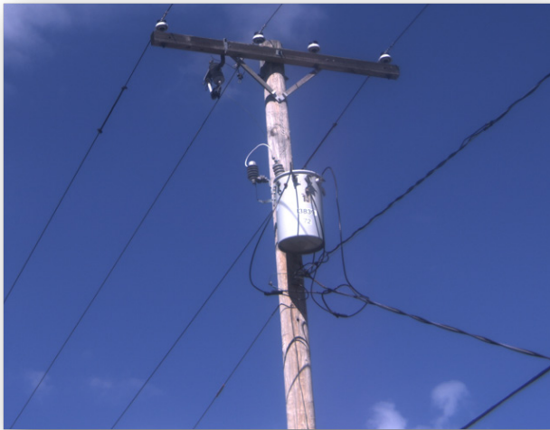
Figure 6: FirstEnergy asset identification from a single Sr Edge photo
