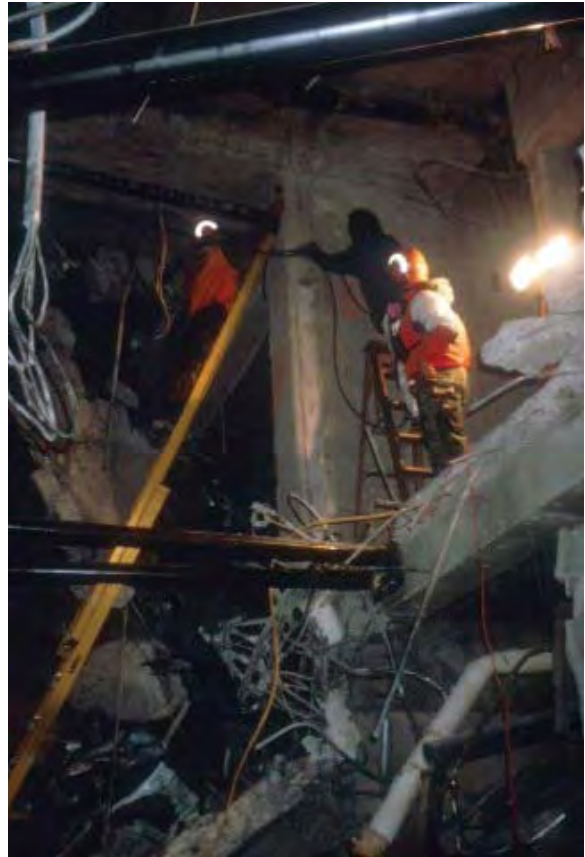
St. Louis District Structure Specialist Tom Niedernhofer conducting inspection at Oklahoma City bombing site
