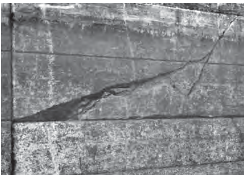
Crack in auxiliary lock wall
