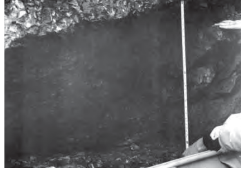
Closeup of crack in lock wall
