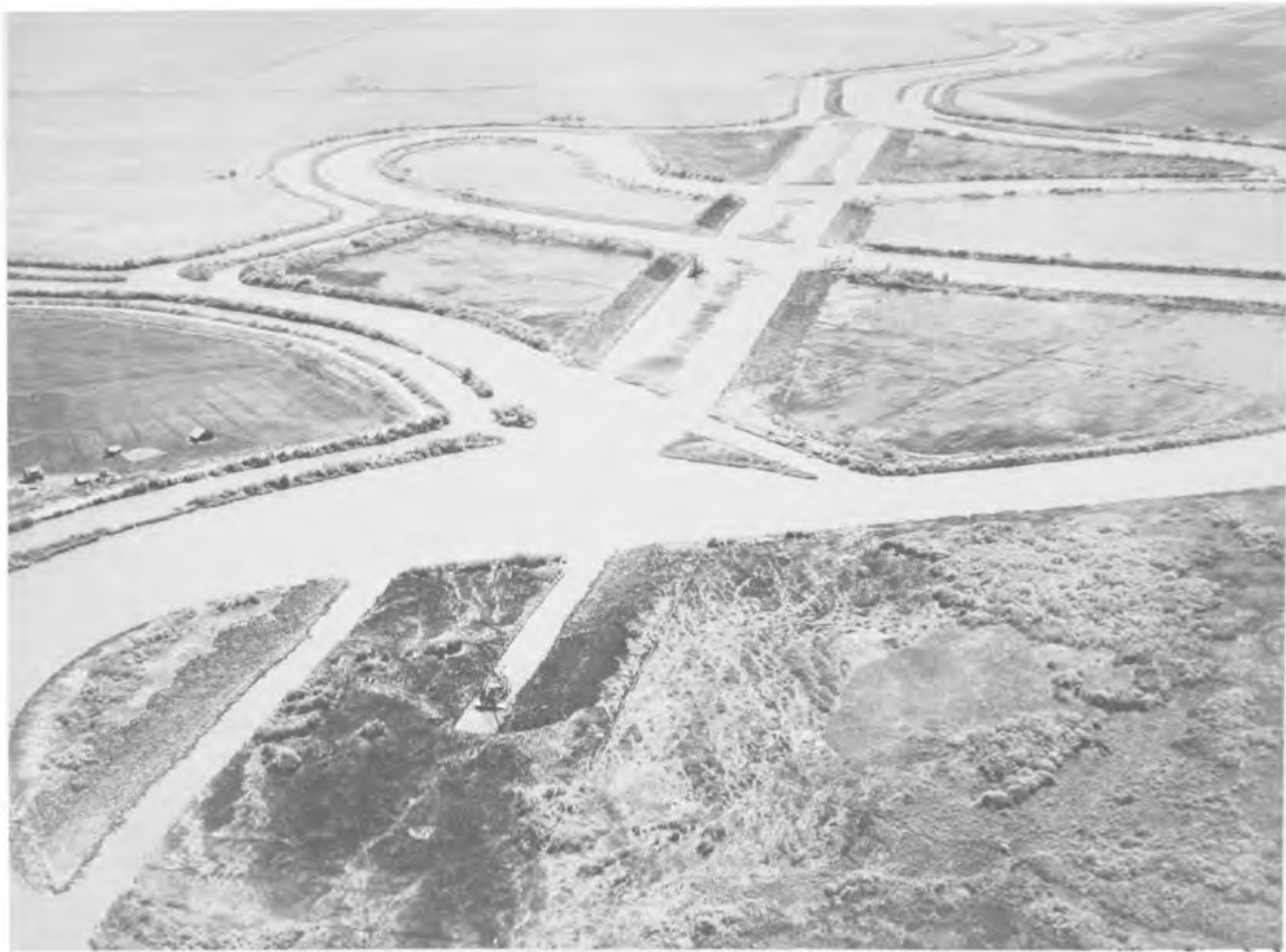
DREDGES HARD AT WORK ON STOCKTON CHANNEL DURING THE EARLY THIRTIES. (Army Corps of Engineers Photo)
