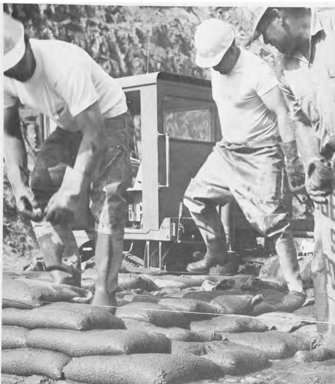
PLACING CONCRETE-FILLED SANDBAGS ACROSS THE LIP OF THE TERMINUS DAM SPILLWAY, THE SACRAMENTO DISTRICT, US ARMY CORPS OF ENGINEERS, GAINED ABOUT 10,000 ACRE-FEET OF ADDITIONAL STORAGE SPACE DURING THE RECORD SNOWPACK SNOWMELT OF JUNE 1969.
