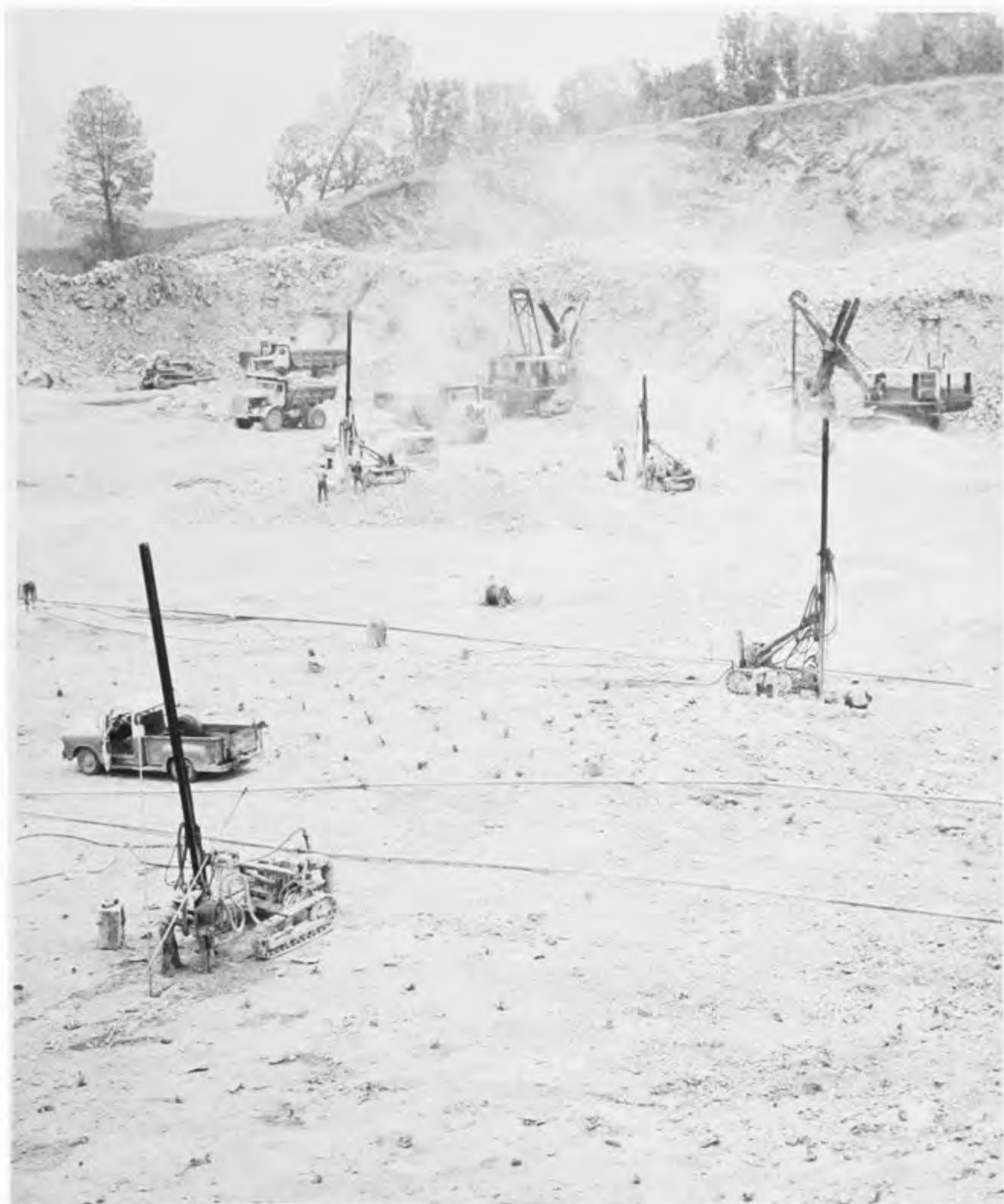
BORROW PIT AT NEW HOGAN DAM SITE — PHOTO TAKEN IN EARLY 1964. (Army Corps of Engineers Photo)
