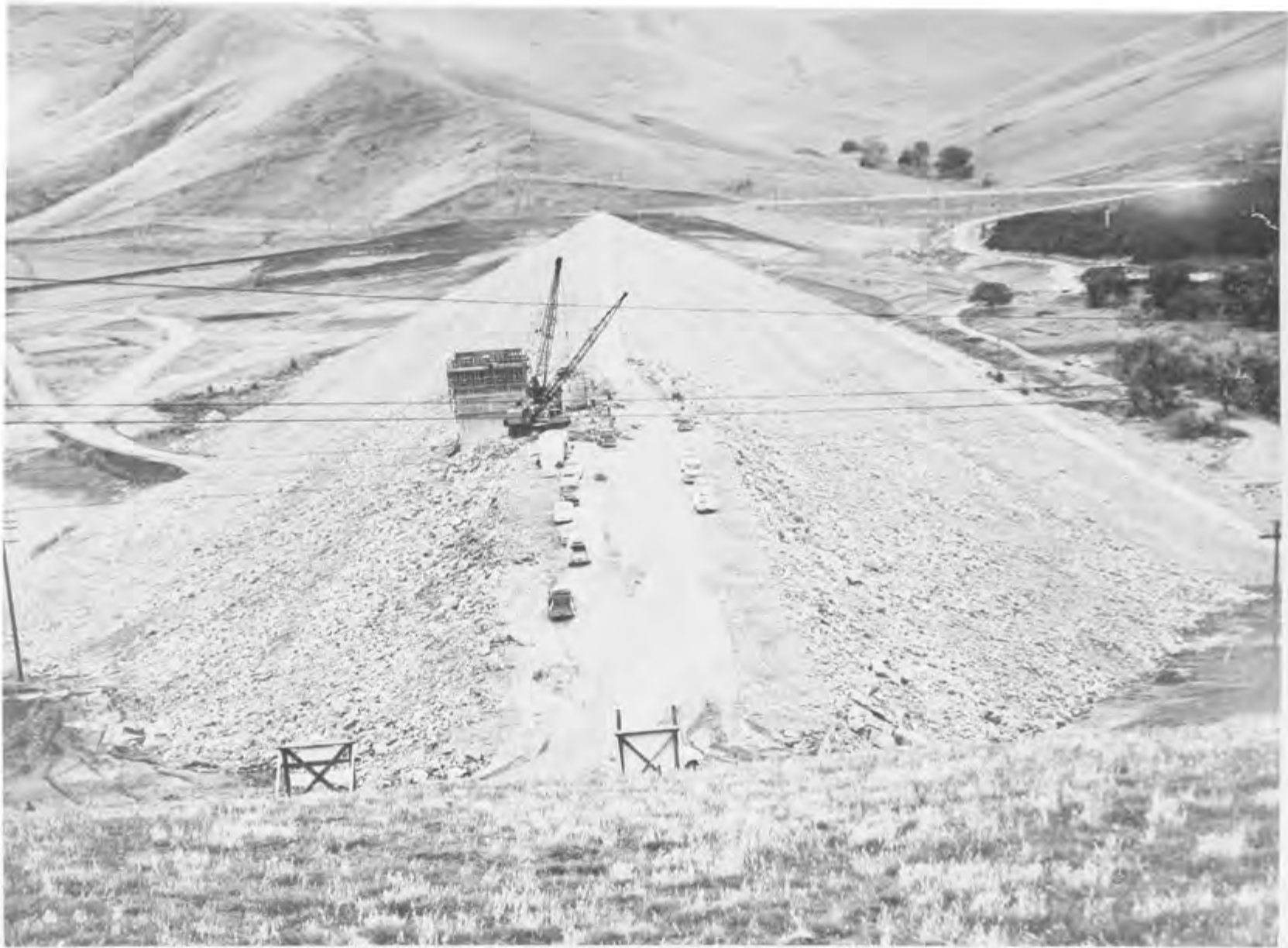
SUCCESS DAM — NEARLY COMPLETE: NOTE THE CONTROL TOWER ON THE LEFT. (Army Corps of Engineers Photo)
