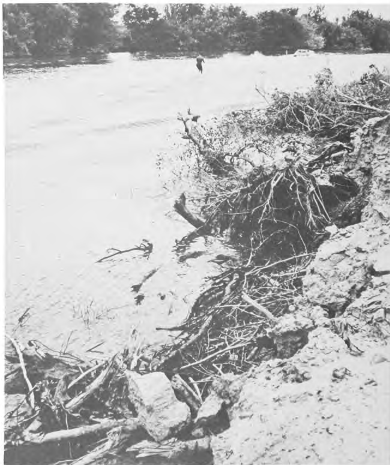
A GRAPHIC EXAMPLE OF LEVEE EROSION ATTRIBUTABLE, IN EVER-INCREASING CASES, TO THE WAVE ACTION PRODUCED BY BOATS AND WATER SKIERS.
