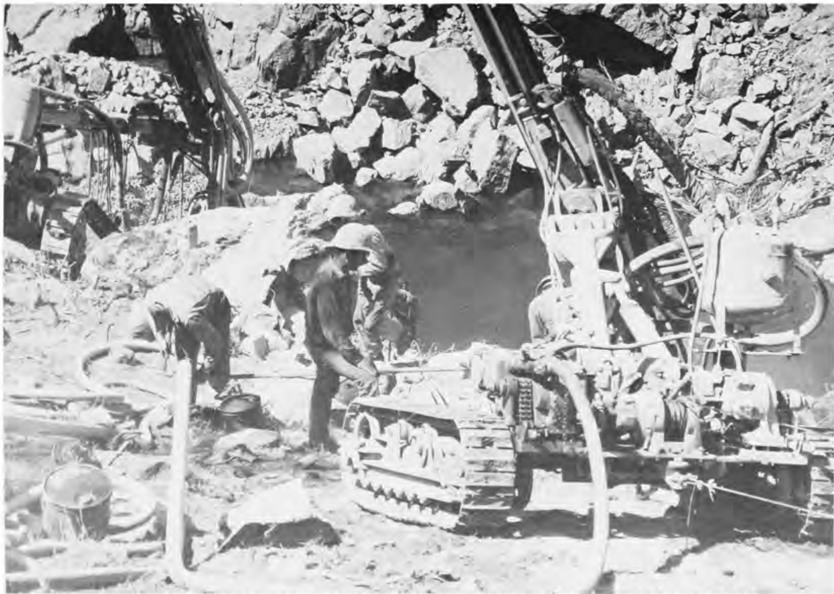
OUTLET (DOWNSTREAM) PORTAL OF THE DIVERSION TUNNEL UNDER CONSTRUCTION AT NEW MELONES DAM PROJECT. THIS TUNNEL WILL DIVERT STANISLAUS RIVER WATER AROUND THE DAM CONSTRUCTION SITE.
