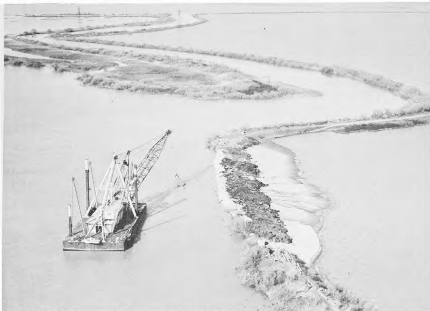
EMERGENCY LEVEE REPAIR WORK — SHERMAN ISLAND IN THE SACRAMENTO-SAN JOAQUIN DELTA — 13 FEBRUARY 1969.
