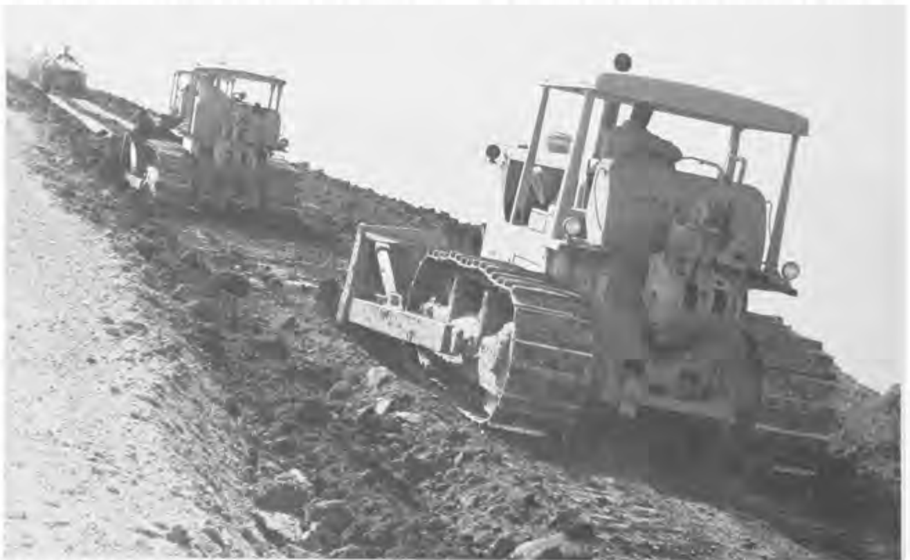
A CONVOY OF DOZERS RAISE A LEVEE IN THE FLOODED TULARE LAKE BASIN TO PROTECT CROPS FROM BEING DESTROYED. THE BASIN RECEIVED BOTH RAINFLOOD AND SNOWMELT WATER FROM ONE OF THE WETTEST SEASONS IN HISTORY IN THE HIGH SIERRA NEVADA. APRIL 1969.
