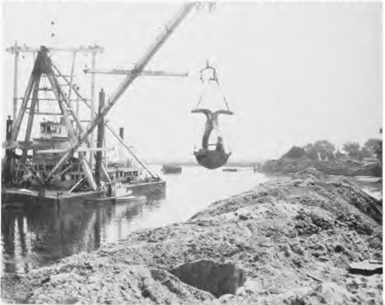
WORK CONTINUED ON STOCKTON CHANNEL THROUGHOUT THE GREAT DEPRESSION. (Army Corps of Engineers Photo)
