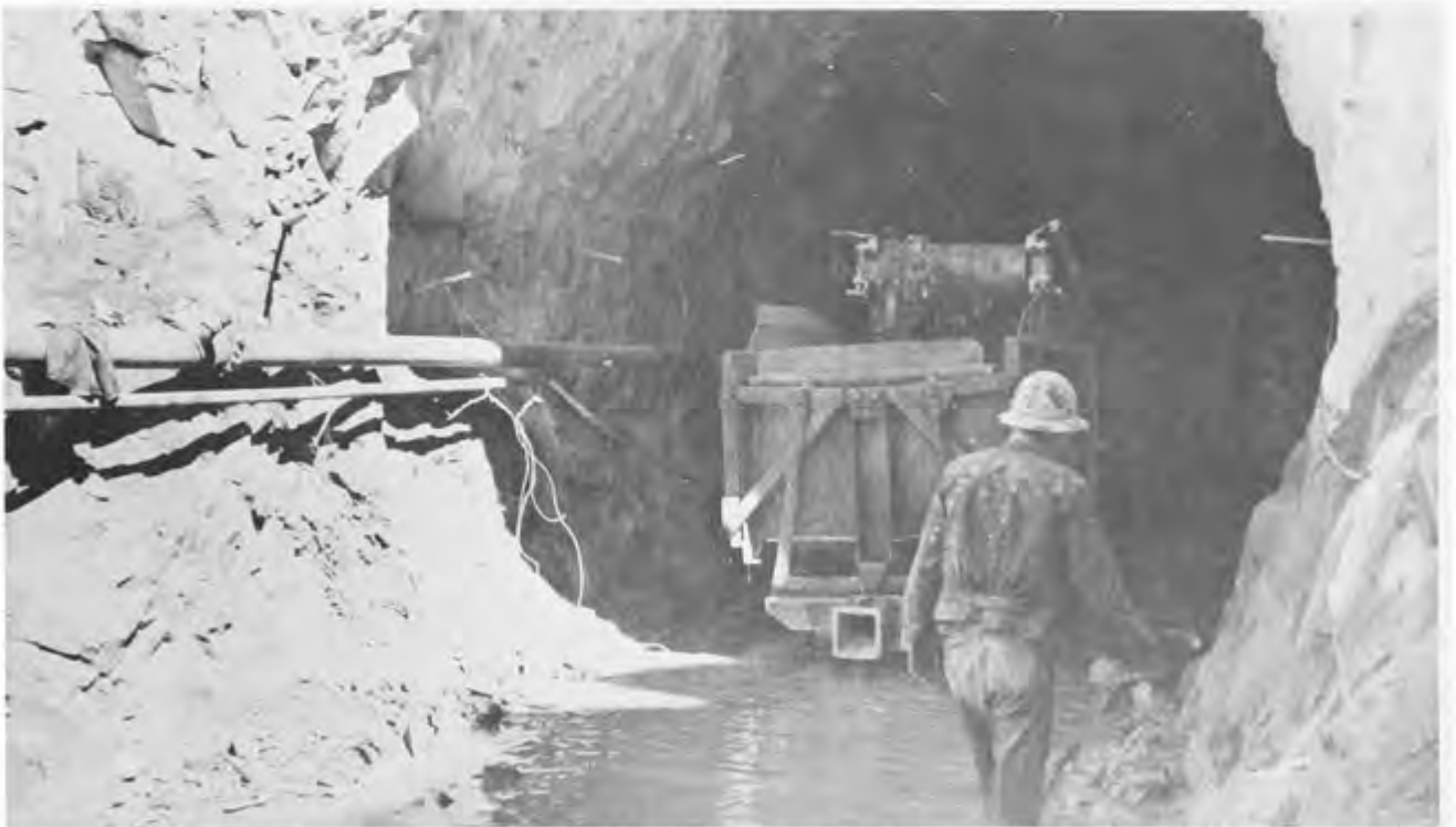
CONSTRUCTION OF THE OUTLET TUNNEL — ISABELLA DAM ON THE KERN RIVER — 1950. (Army Corps of Engineers Photos)
