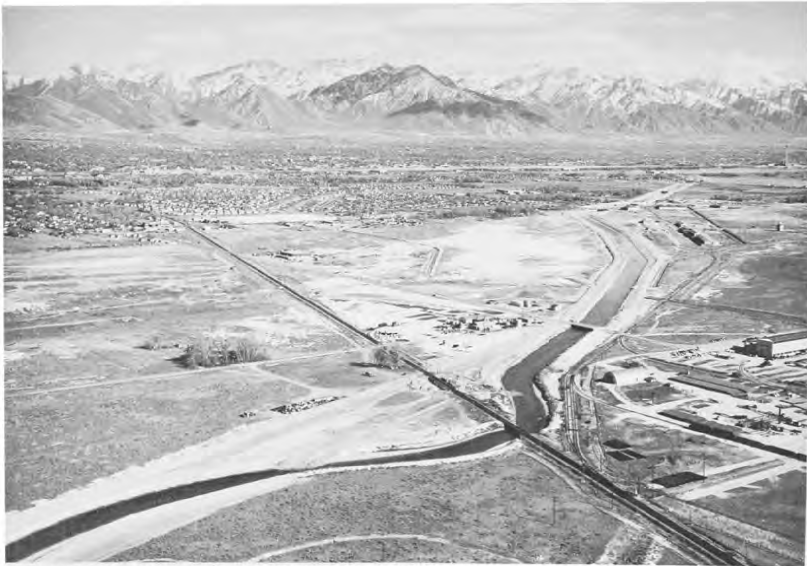
LEVEE CONSTRUCTION AND CHANNEL IMPROVEMENT, JORDAN RIVER, SALT LAKE CITY, UTAH. SURPLUS CANAL REALIGNMENT AND NEW RAILROAD BRIDGE ON U.P. RAILROAD LINE, LOOKING SOUTHEAST. APRIL 1960
