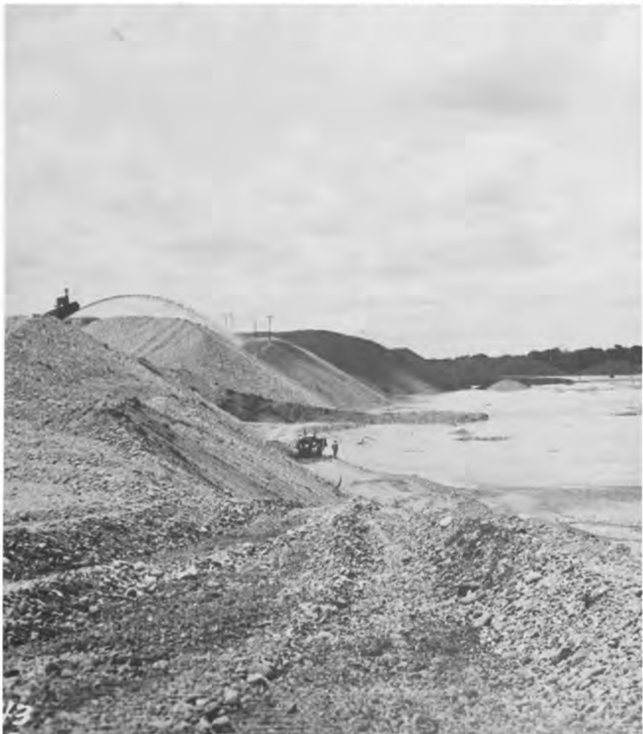
TRAINING WALLS NEAR DAGUERRE POINT DAM, DESIGNED TO HELP KEEP THE YUBA RIVER UNDER CONTROL.
