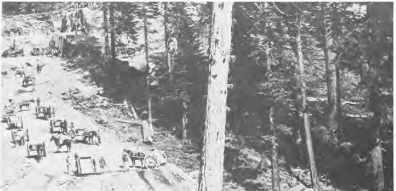
CHINESE LABORERS WORKING WITH PICKS AND SHOVELS AND DUMP CARTS BUILDING THE EMBANKMENT AND MAKING A CUT (MATERIAL FROM WHICH WAS USED TO FILL THE BANK) AT SAILOR'S SPUR, 80 MILES FROM SACRAMENTO IN 1866. IN THE BACKGROUND IS AN EXCELLENT EXAMPLE OF CENTRAL PACIFIC'S SHELF-GRADING METHOD IN WHICH DIFFERENT TEAMS OF MEN WORKED ON DIFFERENT LEVELS TO SPEED THE WORK TO COMPLETION.
