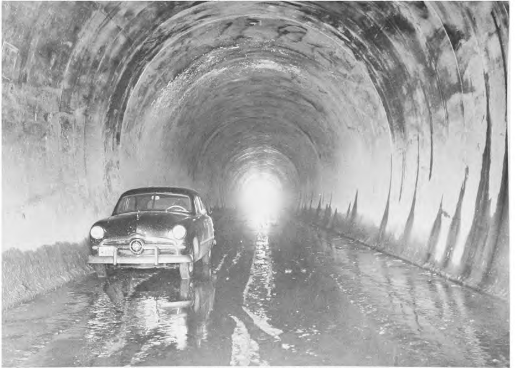
FOLSOM DAM PROJECT NEAR FOLSOM, CALIFORNIA. VIEW OF DIVERSION TUNNEL LOOKING DOWNSTREAM FROM STA. 6+55 ON RIGHT ABUTMENT OF MAIN DAM.
