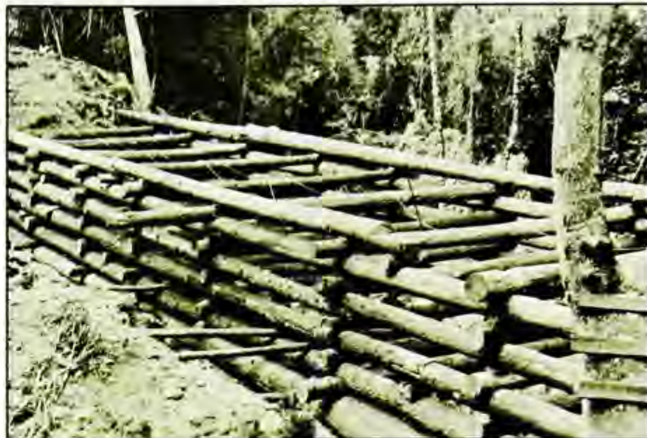
Crib work for a new dam to store debris of the Crusade Mine, 1933. (Corps of Engineers' photo)
