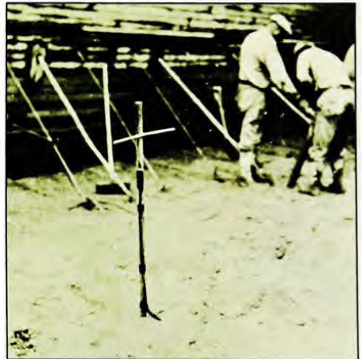
Resistance thermometer installation after cable grooves on top of pour were filled with grout (10/28/38).
