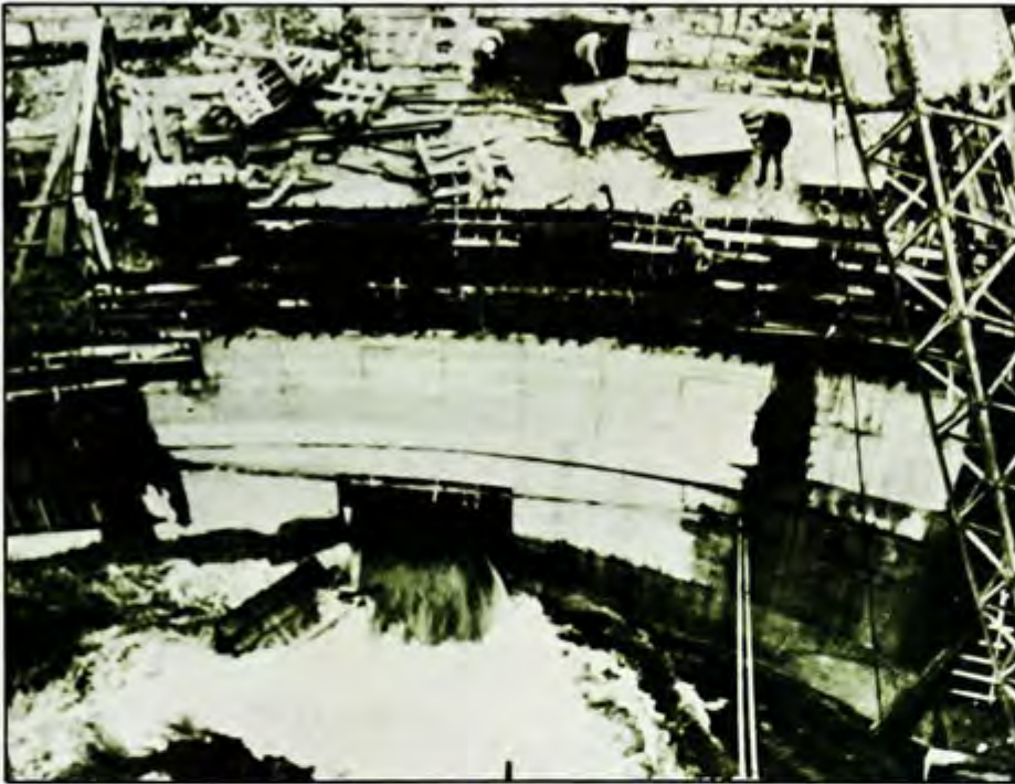
General view of cable recesses on downstream face of dam, showing cable recess above river diversion work (11/3/38).
