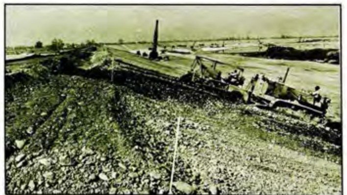
Corps of Engineers crews repair levees near Yuba City following the disastrous flood of 1955. (Corps of Engineers' photos)
