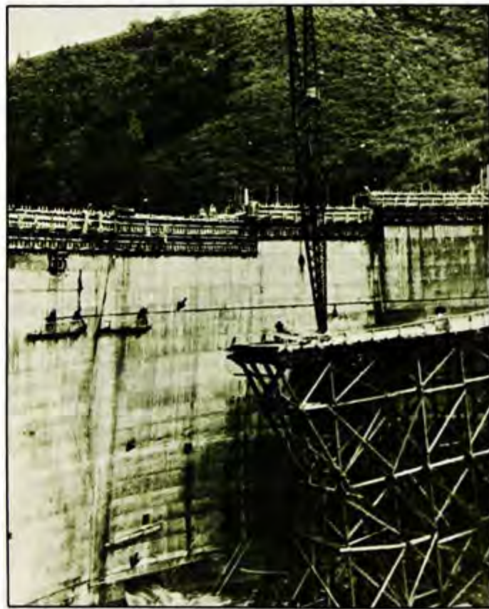
Arrows indicate cable recesses on downstream face of dam. Workmen are drypacking upper cable recesses.
