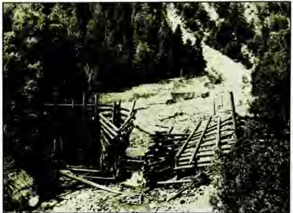
Log dam failure, Volcano Canyon near Foresthill
