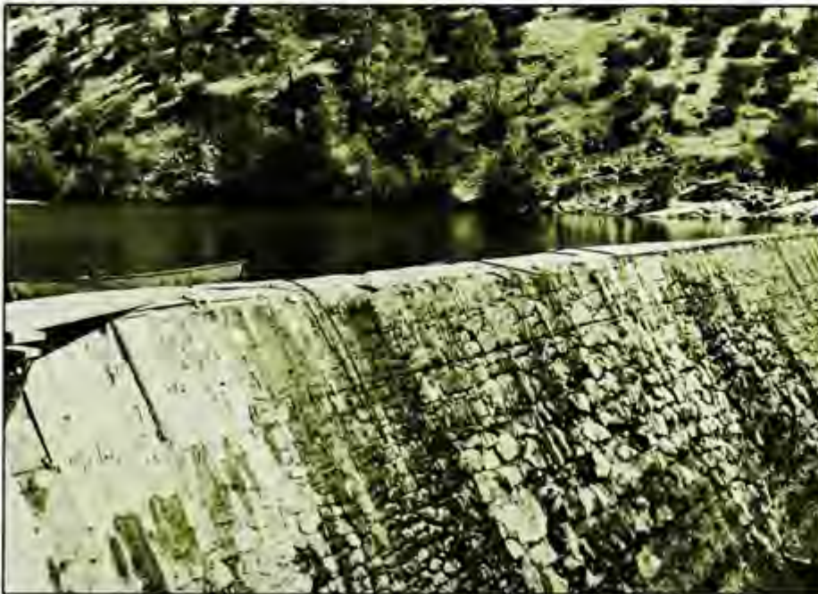
Stone Dam, the type that Mendell felt could restrain mining debris. (Corps of Engineers' photo)
