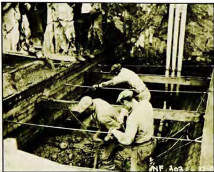
Left abutment of dam. Note 3½" conduits for strain meter cables (3/23/38). Above shows something of the foundation material of the left end of dam now hidden by retaining wall.
