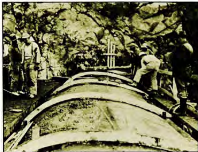
Finishing spillway crest in block 13 at elev. 718 (12/23/38). The rock in the upper right hand corner was involved in the landslide during the spring of 1940.
