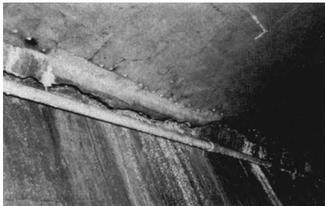
Figure 2-11. Isolated crack caused by structural overload
