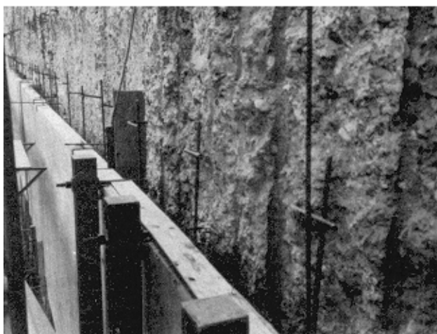
Figure 8-15. Installation of precast concrete stay-in-place forms at Troy Lock, Hudson River (Miles 1993)
