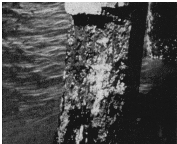
Figure 2-13. Disintegration of concrete caused by exposure to acidic water
