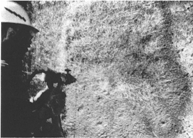
a. Applying the coating with equipment that simultaneously sprays the mortar from one nozzle while it chops and blows the fiber from a cutterhead
