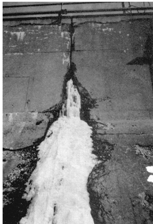
Figure 2-28. Water seepage through joint
