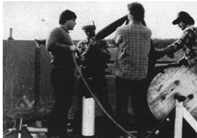
Figure 8-23. Two-component natural rubber and elastomer coated nylon sleeve being inserted into drill hole, Bagnell Dam
