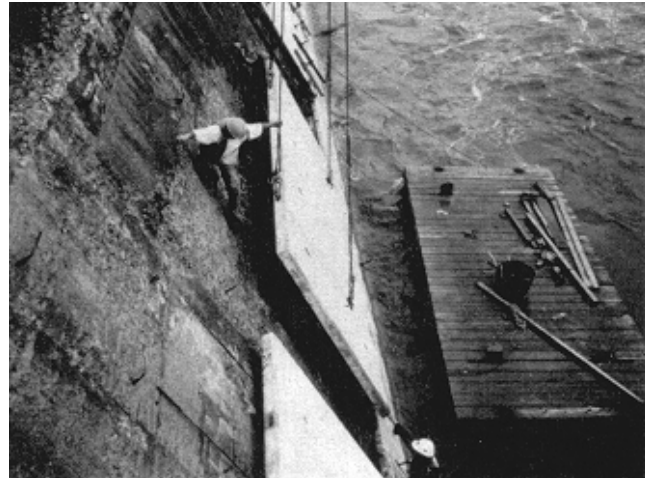
Figure 8-17. Installing precast concrete panels used to overlay the back side of the river wall at Troy Lock, Hudson River (Miles 1993)
