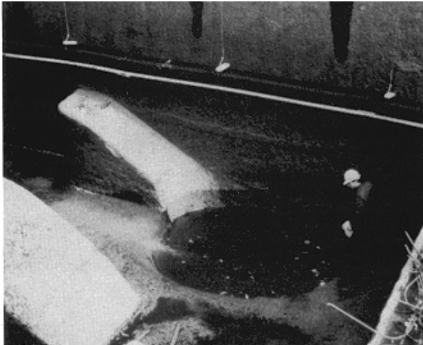
a. Scour holes behind baffles
