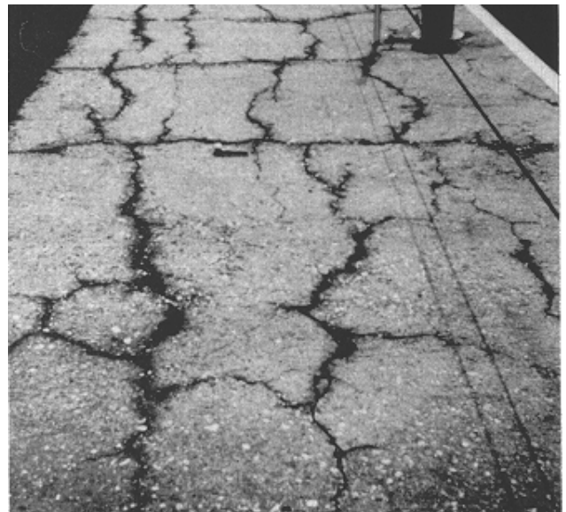
Figure 2-6. Pattern cracking resulting from alkali-silica reaction
