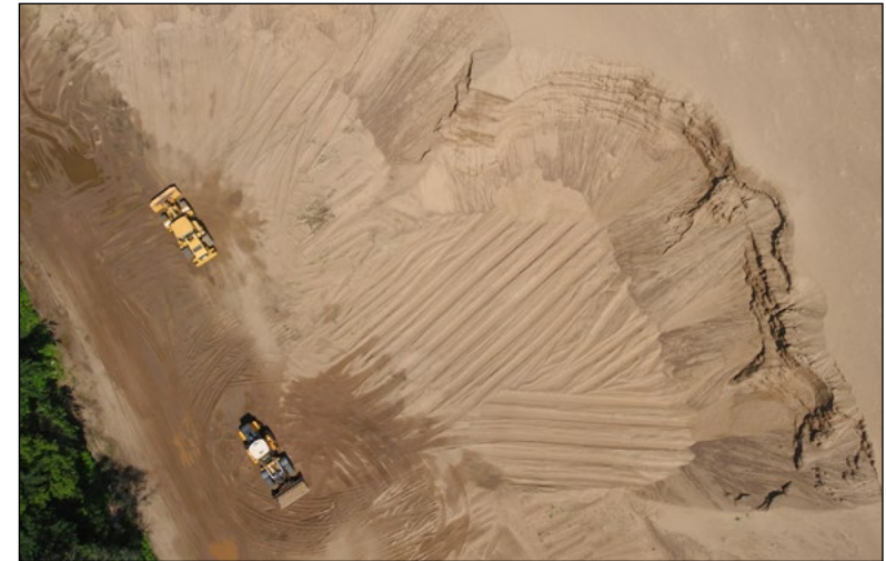
Small unmanned aircraft imagery of the Wabasha gravel pit from 390 feet above ground level, near Wabasha, Minnesota, June 30. USACE unmanned aircraft imagery
