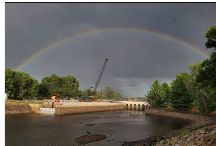
A rainbow over the Sandy Lake Dam rehabilitation near McGregor, Minnesota, June 8. USACE photo by Noah Brown
