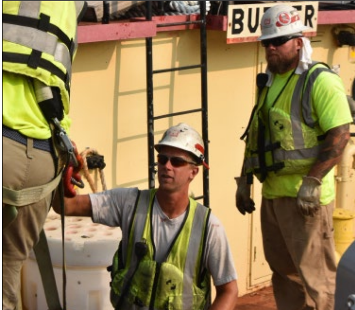
Scott Rolbiecki and Nick Stanton, maintenance and repair, work on the miter gate replacement at Lock and Dam 2, near Hastings, Minnesota, July 20. USACE photo by George Stringham
