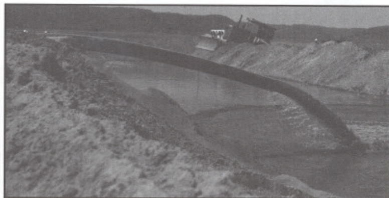
In the foreground, dredged fill material flows into a catch basin as it builds up an island near Stoddard, Wis.
