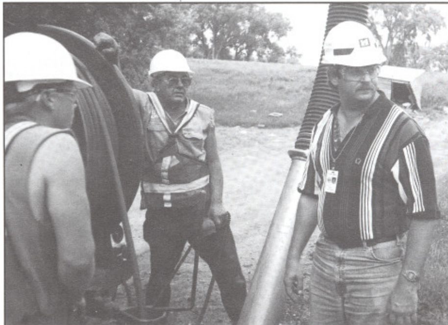
Photo by Burch Communications
