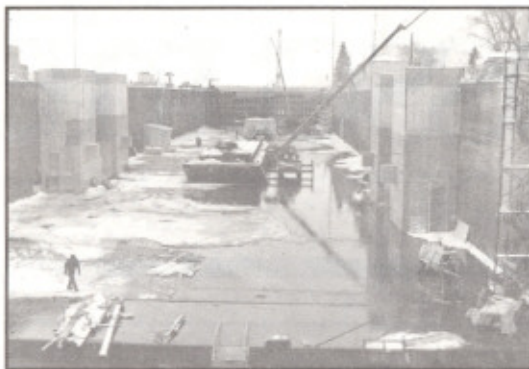
The St. Paul District drained Lock and Dam No. 8 at Genoa, Wisconsin for rehabilitation and maintenance in December 1991. The
