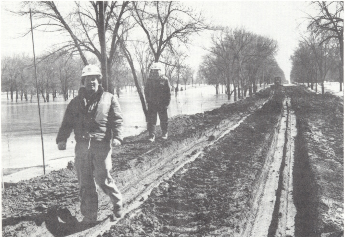
Dick Martig of the Rochester Resident Office (left) and Jeff McGrath, economist in Planning Division, walk the 800-foot levee under construction along Belmont Avenue in Grand Forks, North Dakota. Corps contracts for this project called for 10,000 yards of dirt to construct the 10-foot high levee, protecting a residential neighborhood. Total cost was $48,000.
