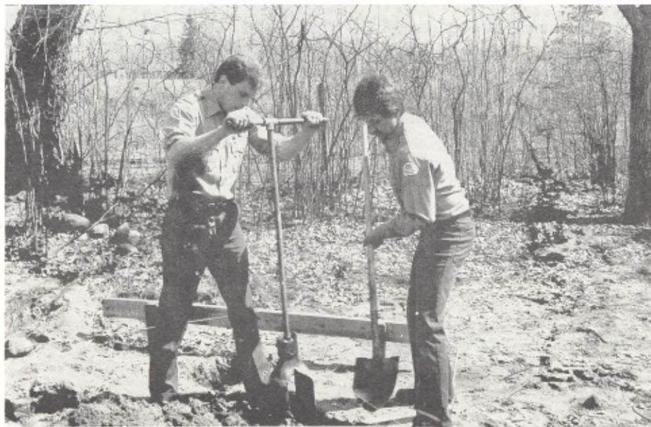
Facilities improvement has been taking place at other District lakes as well. Pictured here are Park Rangers Timm Rennecke and Pat Duffney beginning work on a wooden shelter for firewood storage in the Pokegama Lake campground. Digging post holes was not the most unpleasant thing to be doing on a beautiful, cool morning in April. An identical shelter was constructed at Lake Winnibigoshish.
