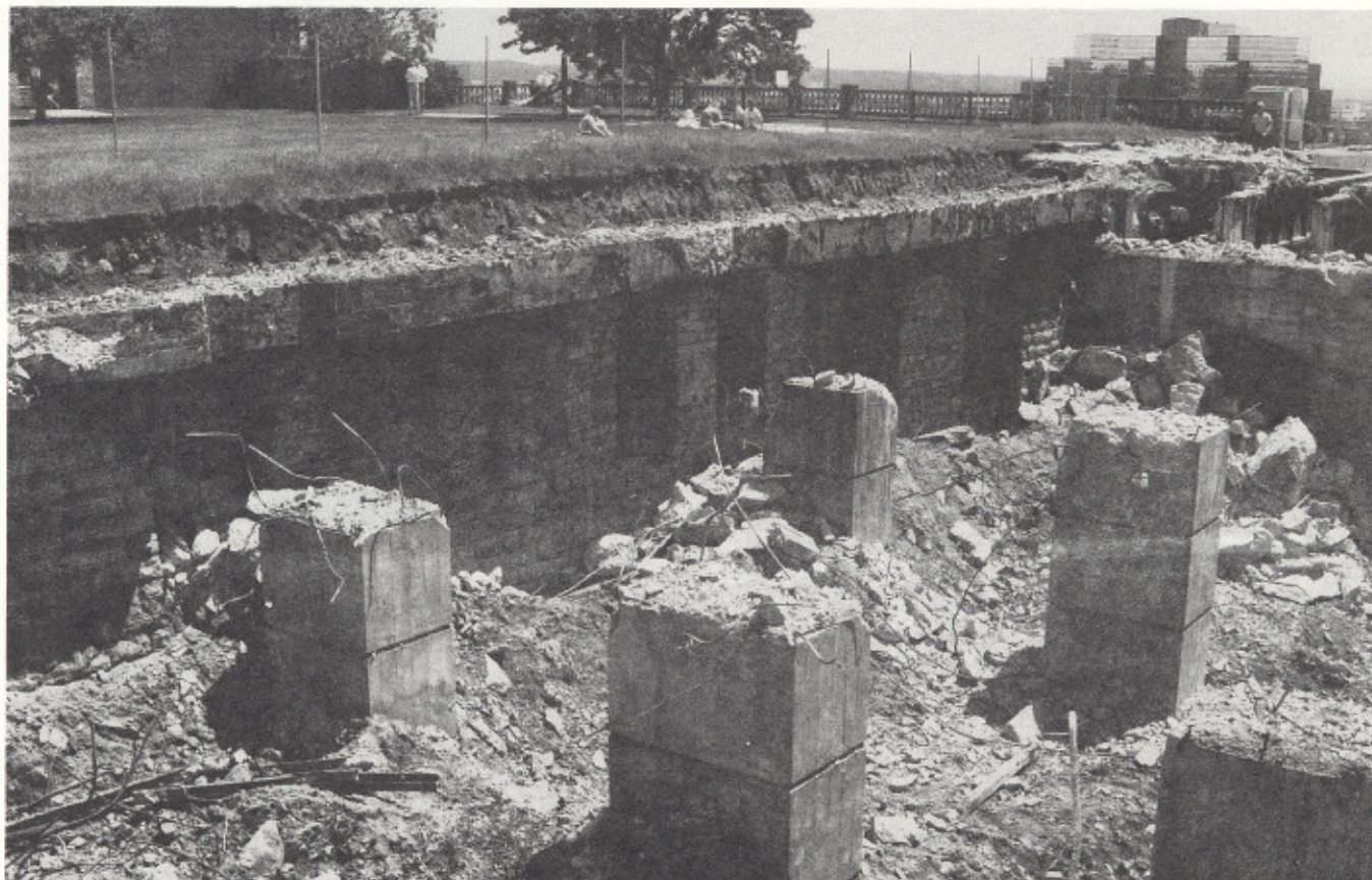
This is the view of the 1881 Army Building's foundations as seen during the Robert Street bridge repair work in June 1989. It shows the same perspective as the circa 1880's cover illustration, except that the top four floors are missing. Note the State Revenue Building in the distance, across the river. The entrance to the American Center building is to the left.
