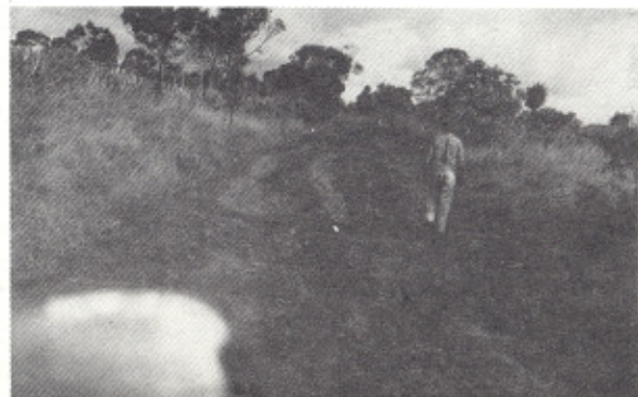
This road surface, with its massive ruts, was the typical road condition found in Tanzania.
