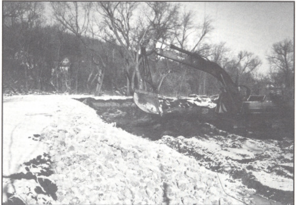
The first stage of the Corps flood control project in Rochester involves excavation and riprapping the riverbank near the mouth of Cascade Creek.
