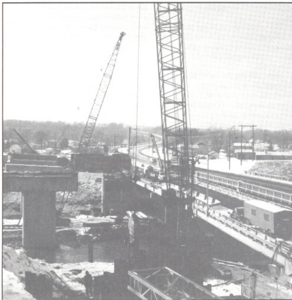
Construction of the Trunk Highway 169 final feature of the Mankato-North Mankato-Le Hillier flood control project.
