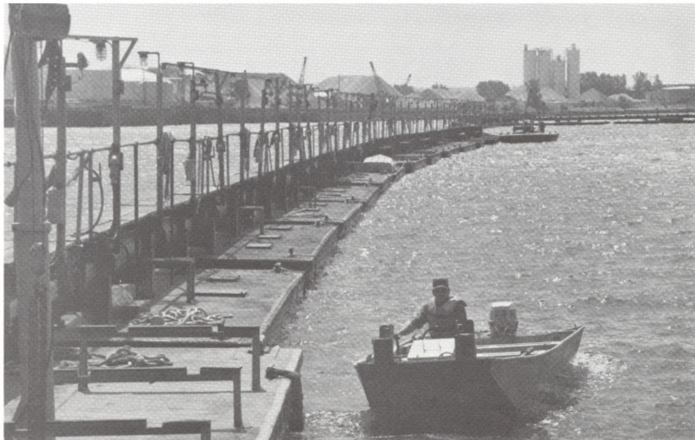
A Texas National Guard member checks the expanse of floating pipeline, which carries the excavated material and water
