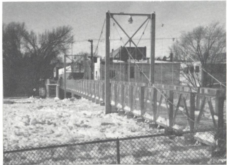
The ice jam at Granite Falls, Minn., along the Minnesota River raised the pedestrian bridge three to six inches off the abutment.
