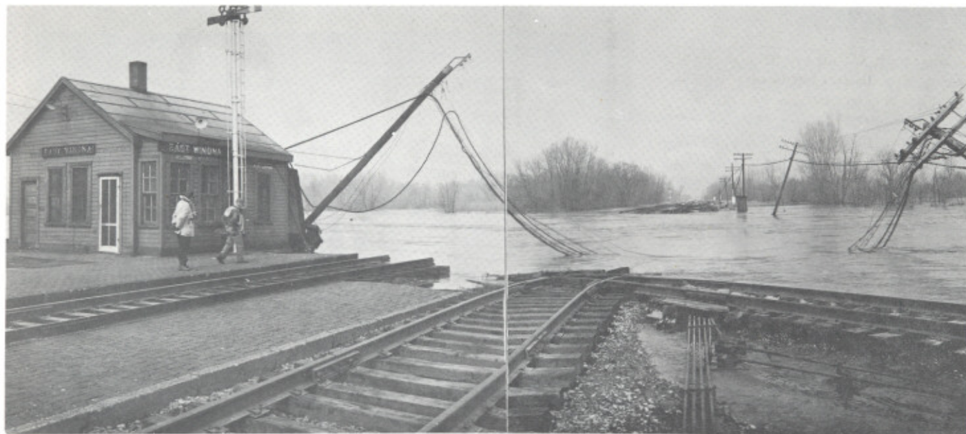
During the 1965 flood on the upper Mississippi River, many bridges and railroad crossings were either flooded or washed away. The photo above shows the washout of railroad tracks and power lines in Winona, Minn.
