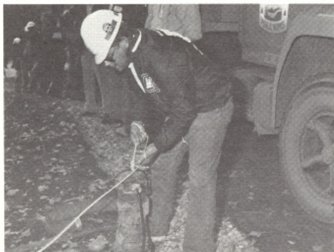
Bruce Ragan prepares a Flygt pump at the Crookston, Minn. flood fight exercise. Photo by Lyle Nicklay
