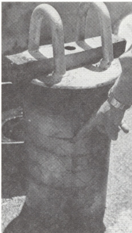
A gudgeon pin removed from the miter gate of Lock and Dam No. 10, shows excessive scouring.
