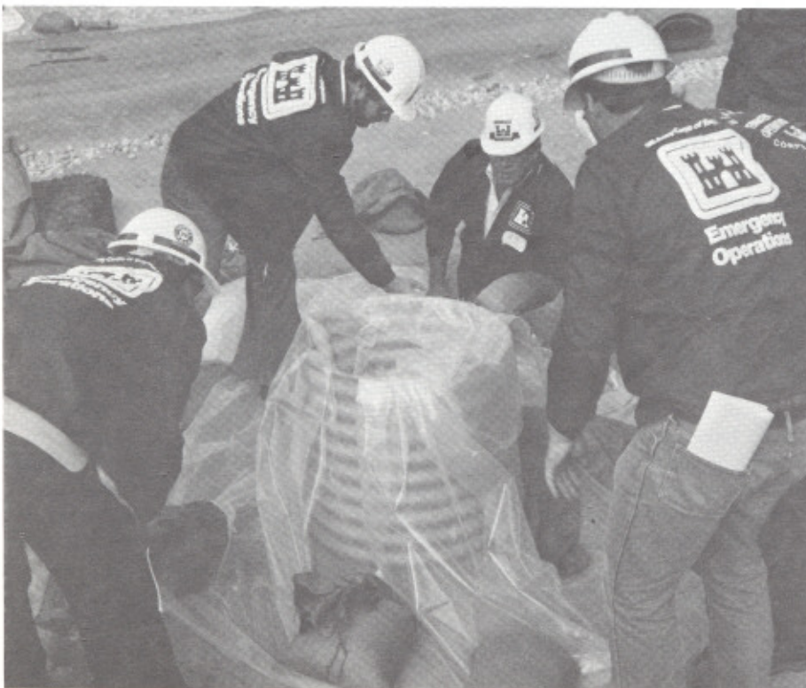
Corps employees place sandbags and poly-sheeting around a CMP to demonstrate protection from a flooding manhole.
