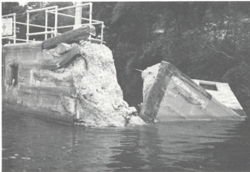
The guidewall lost a piece of concrete 10 by five by six feet in size, and a gage house. (Photo by C. Giaquinto, ED-D)
