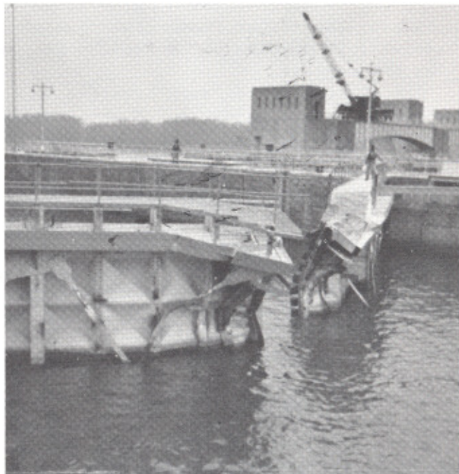
The damaged upper miter gates of Lock 9. (Photo by Carl D. Noel, Lock and Dam 9)
