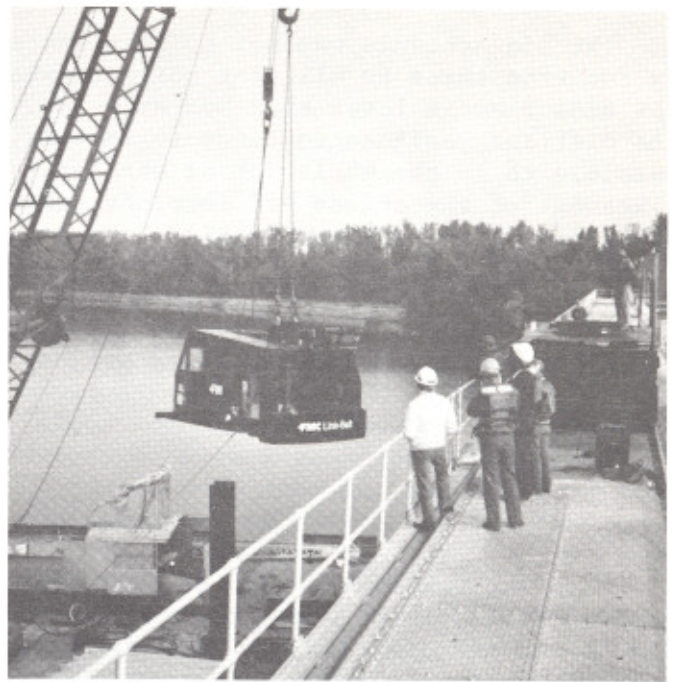
A new crane cab is being hoisted upwards to be placed onto the carriage of the lock facility. The old cab was removed and is on the crane barge (lower left corner). (Photo by Eugene L. Schuppel, Lock and Dam 3)
