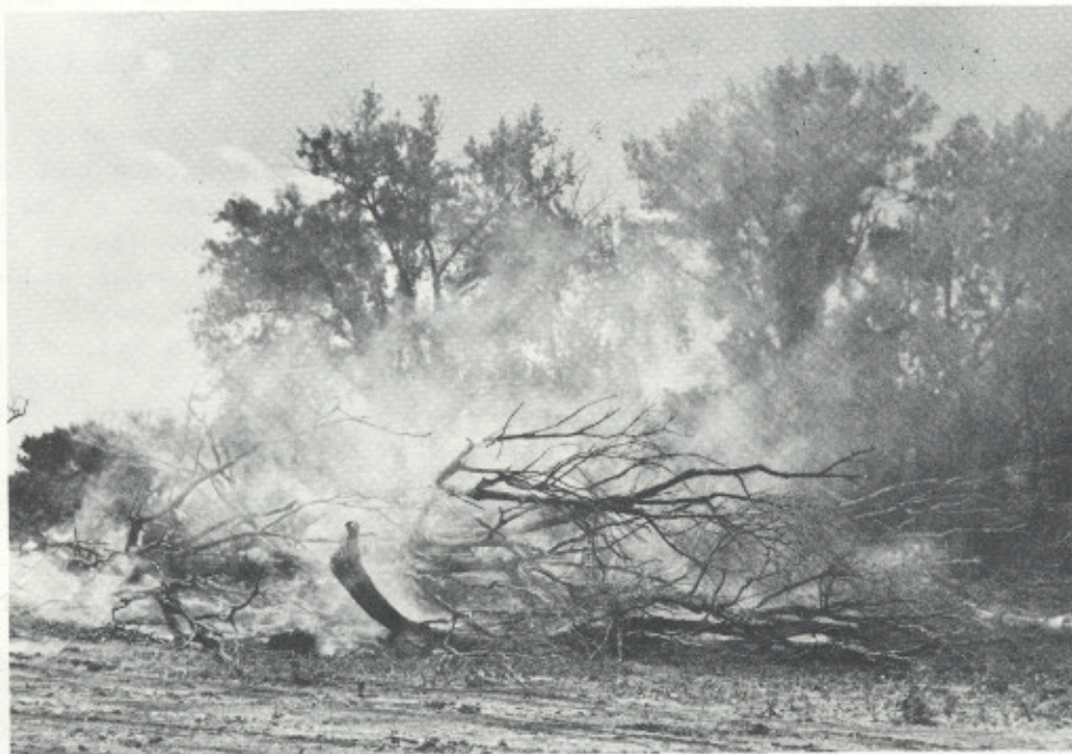
Burning of debris from South Branch during clearing operations. (Photos courtesy of Construction Branch)
