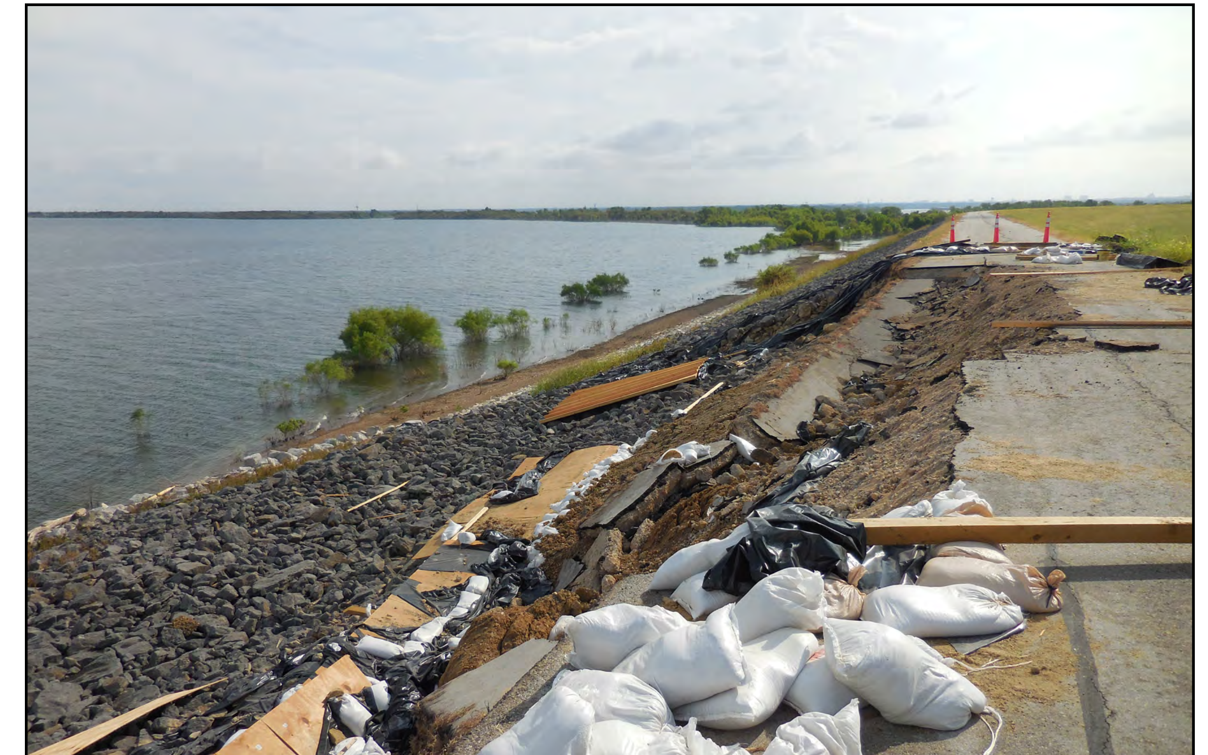
Ongoing repairs to a slide at Lewisville Lake resulting from the May 2015 storms.
