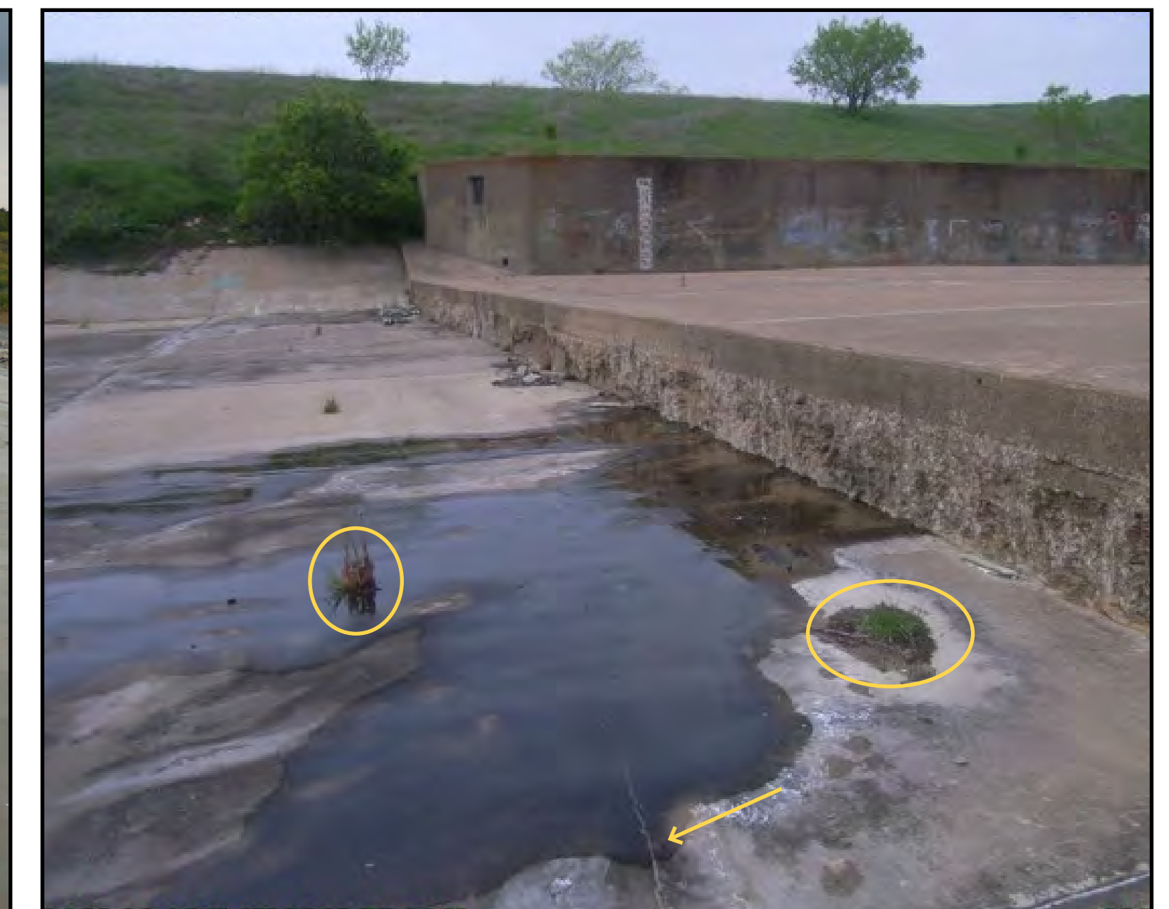
Cracks in the Spillway Apron
