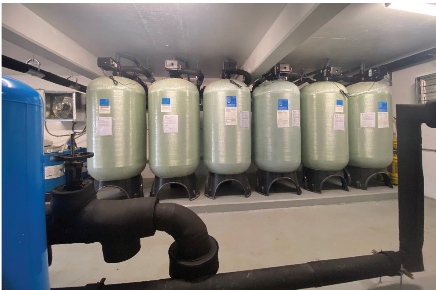
View of GAC tanks area.
