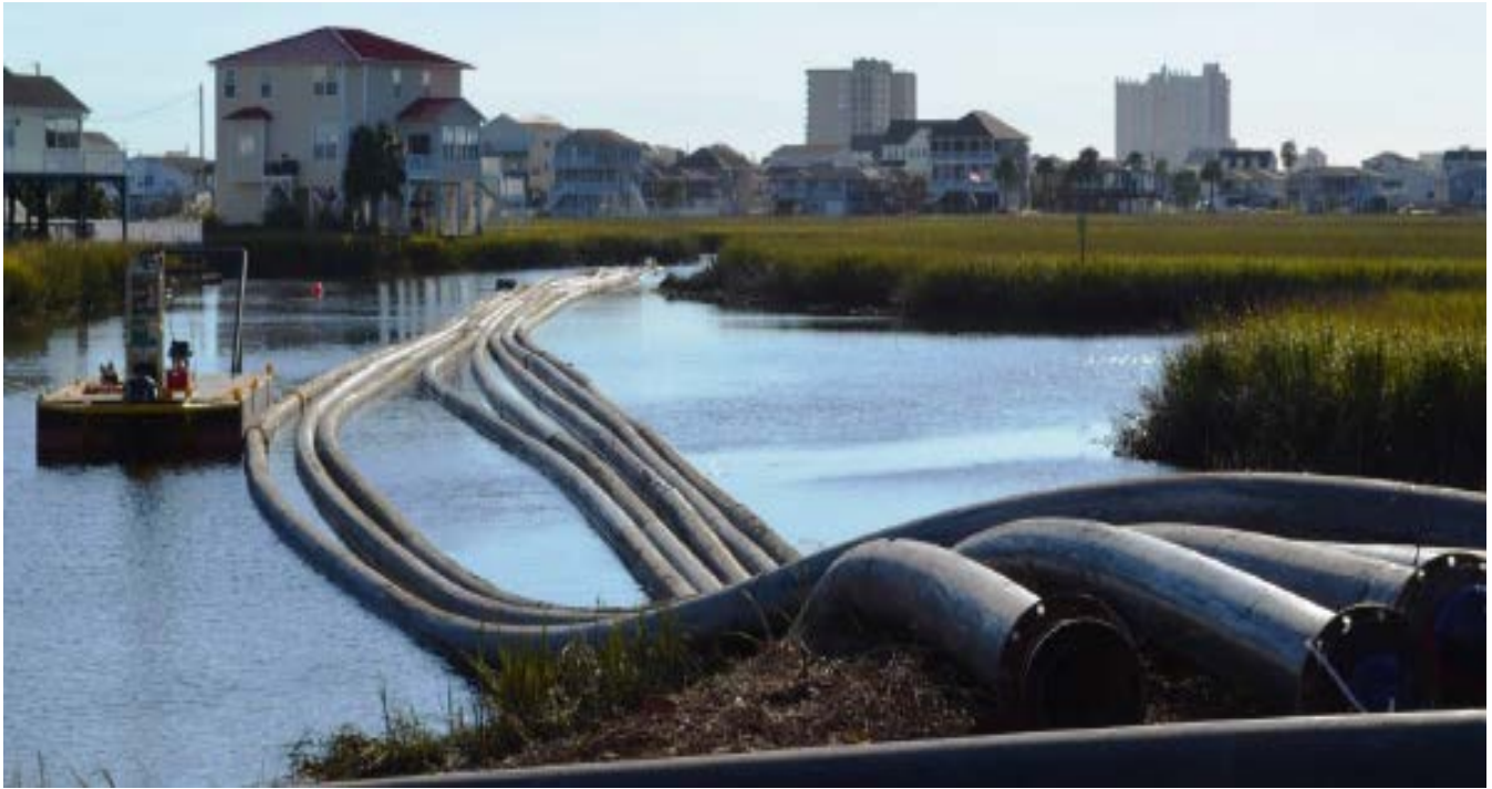
Figure E-2 Pipeline directing dredged material from the project site extending ultimately to the spoils site west of Little River Neck Road.
