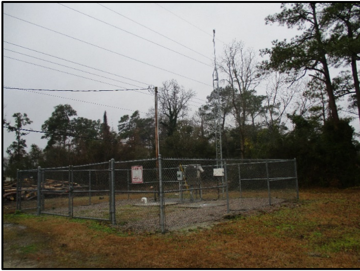
Figure C-2 Typical pump station within the North Myrtle Beach sanitary sewer system
