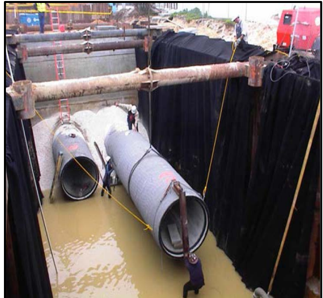
Figure F-3 View of the sediment box and piping of the shoreline section of an ocean outfall project in Myrtle Beach. The large scale nature of this type of stormwater infrastructure project entails significant capital costs.
