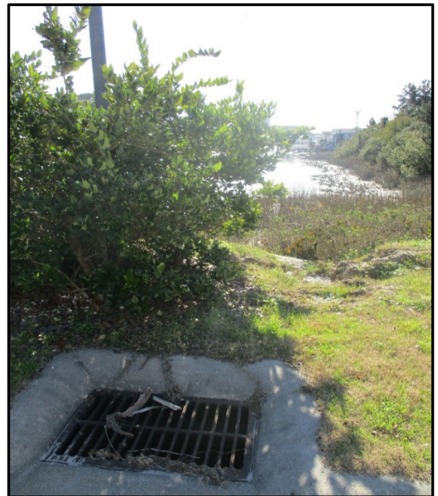
Figure C-6 Typical storm drain adjacent to the Cherry Grove Canal
