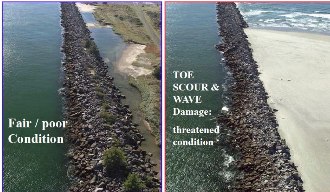
Figure 7. North Jetty Damage Areas
