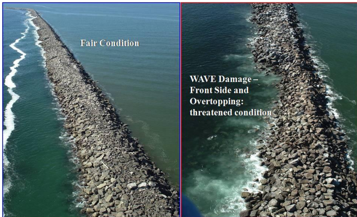
Figure 6. South Jetty Trunk Damage
