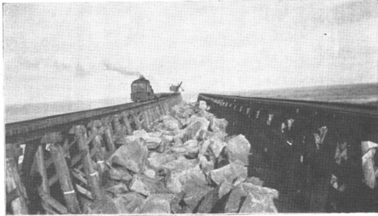
Mouth of Columbia River, Oregon; retopping south jetty; tracks 45 feet between centers; July, 1934.
