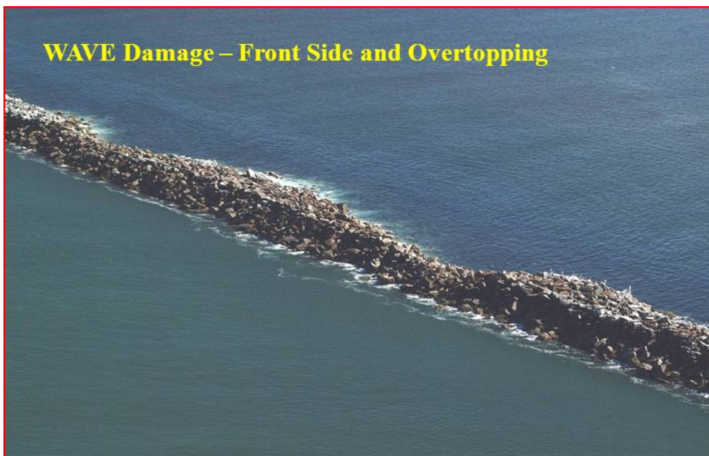
Figure A1- 123. South Jetty Trunk Damage
