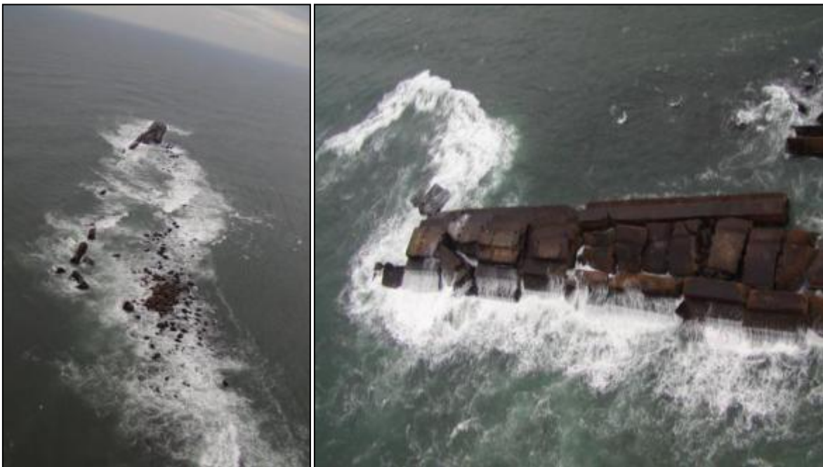
Figure 1-13. Remnant of Concrete Terminal at End of South Jetty
