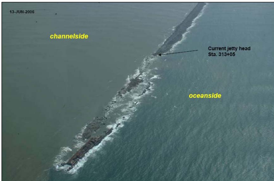
Figure A1- 129. South Jetty Deteriorated Head and Concrete Terminal
