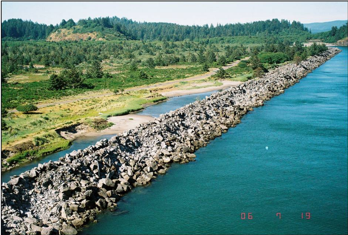
Figure A1- 105. North Jetty Damage Areas
