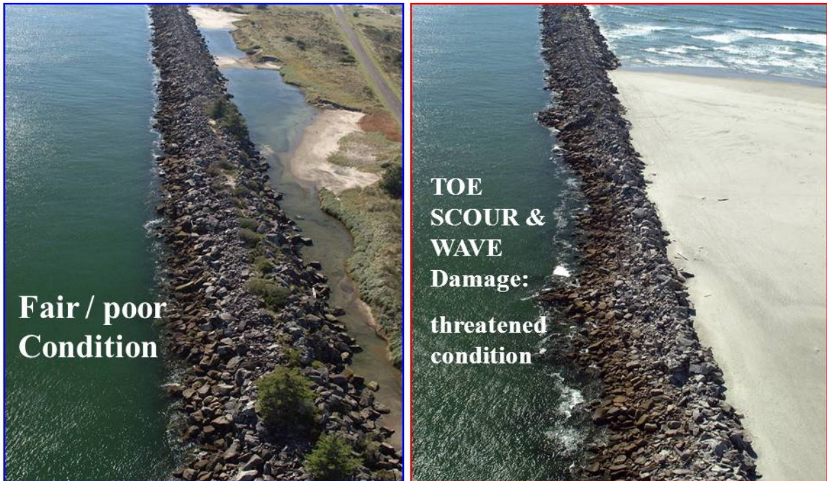
Figure A1- 104. North Jetty Damage Areas
