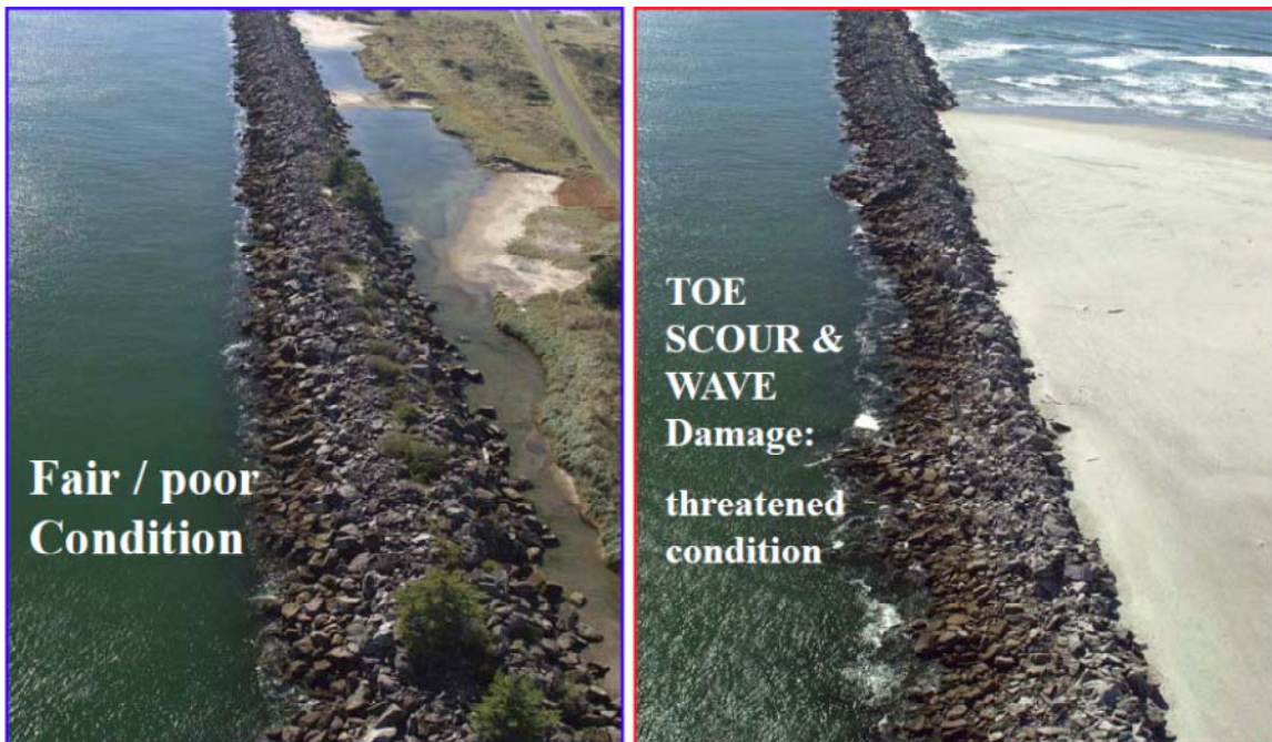
Figure 1-9. North Jetty Damage Areas
