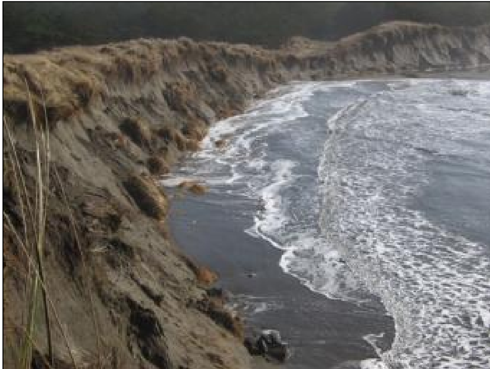
Figure 1-31. Active Shoreline Erosion at the Root of the South Jetty (oceanside)
