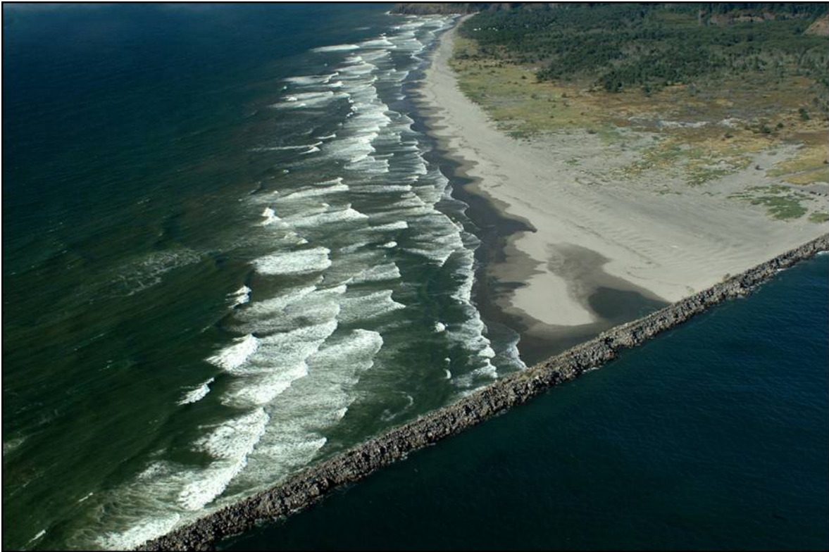
Figure A1- 106. North Jetty Seaward Trunk Damage
