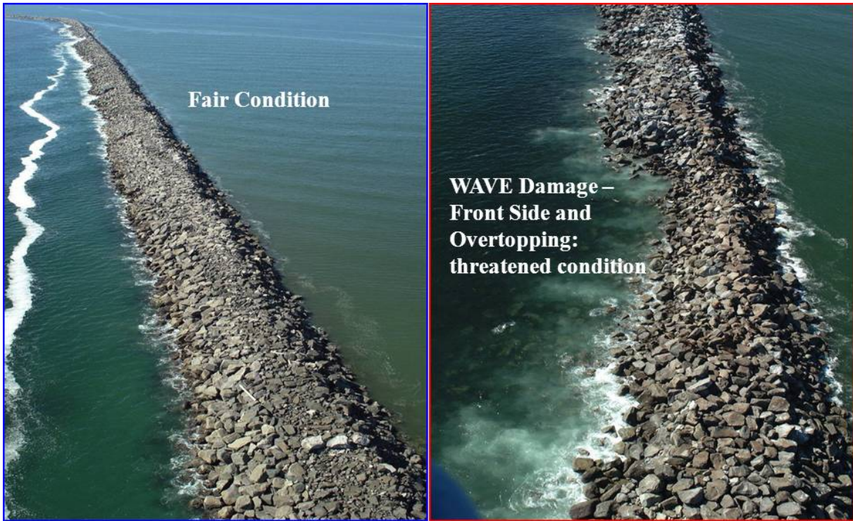
Figure A1- 124. South Jetty Trunk Damage
