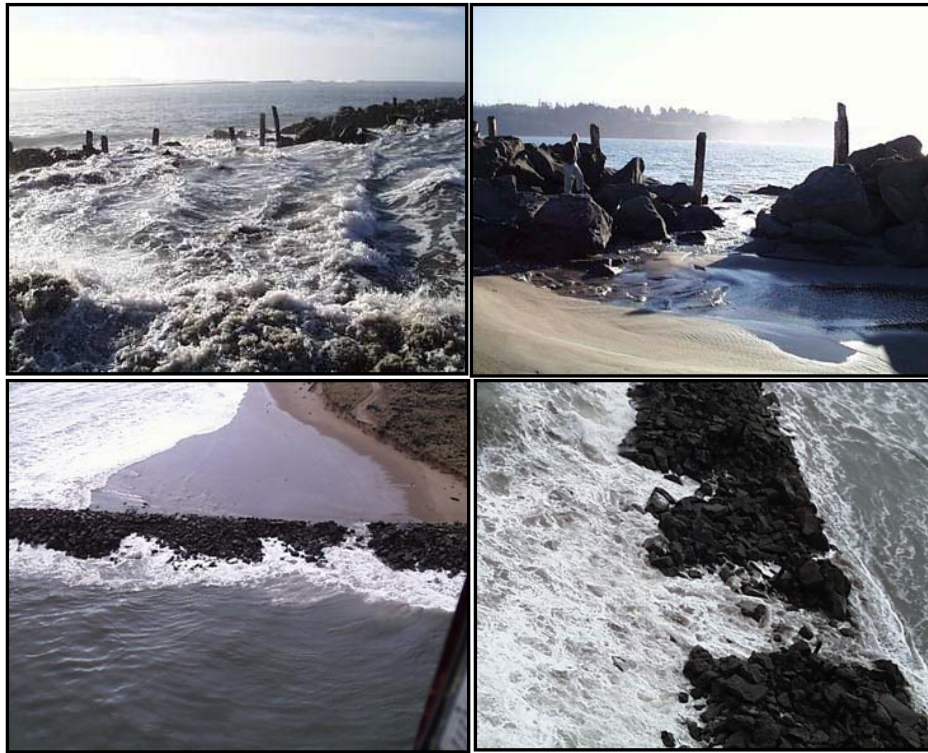
Figure A1- 249. Breached Jetty at Smaller Navigation Entrance
