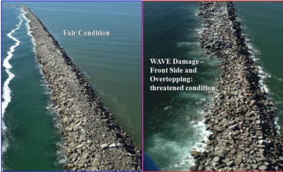
Figure 1-8. South Jetty Damage Areas
