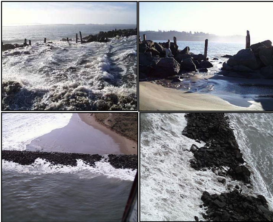
Figure 3-13. Example of a Breached Jetty
