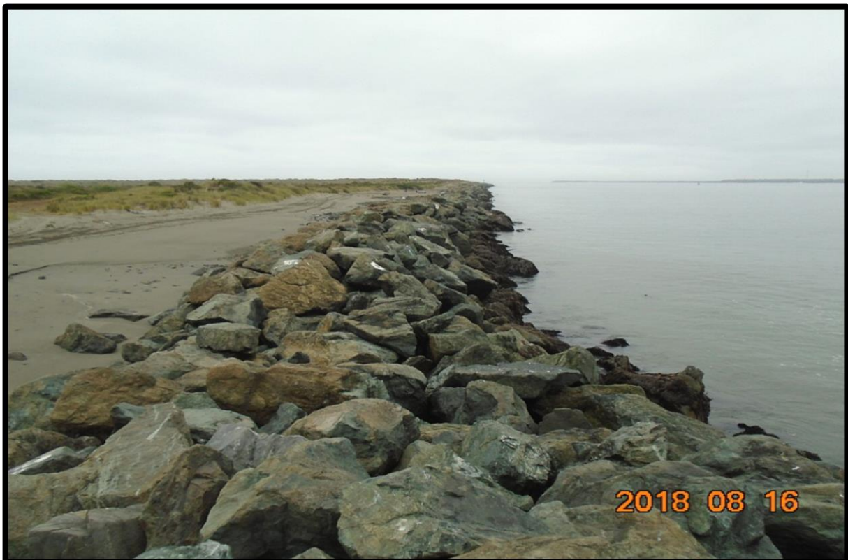
Figure 6. Photo of entire jetty cross-section in need of repair (Type 3).
