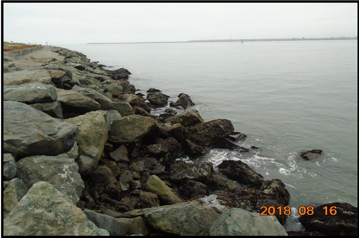
Figure 5. Photo of jetty slope in need of repair (Type 2).
