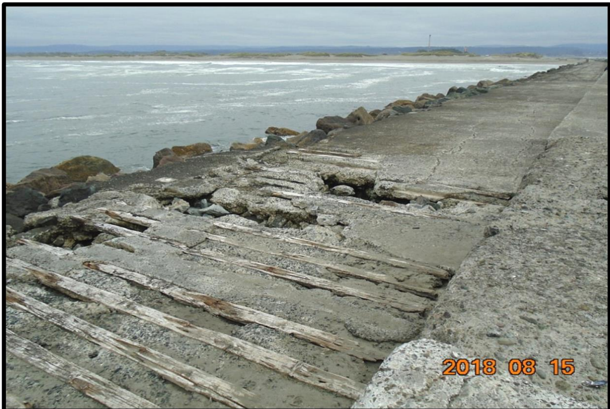
Figure 4. Photo of concrete cap in need of repair (Type 1).
