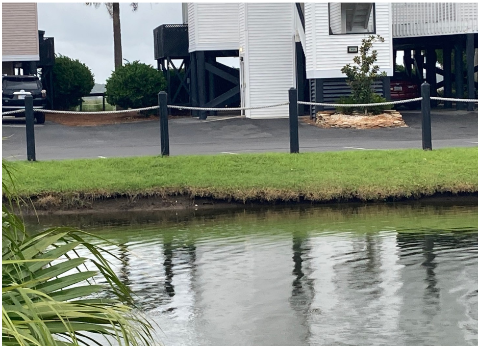
Figure 61: Undercutting of bank observed in a stormwater pond on Edisto Beach without a vegetated buffer between the pond and impervious parking area (photo: A. Scaroni)
