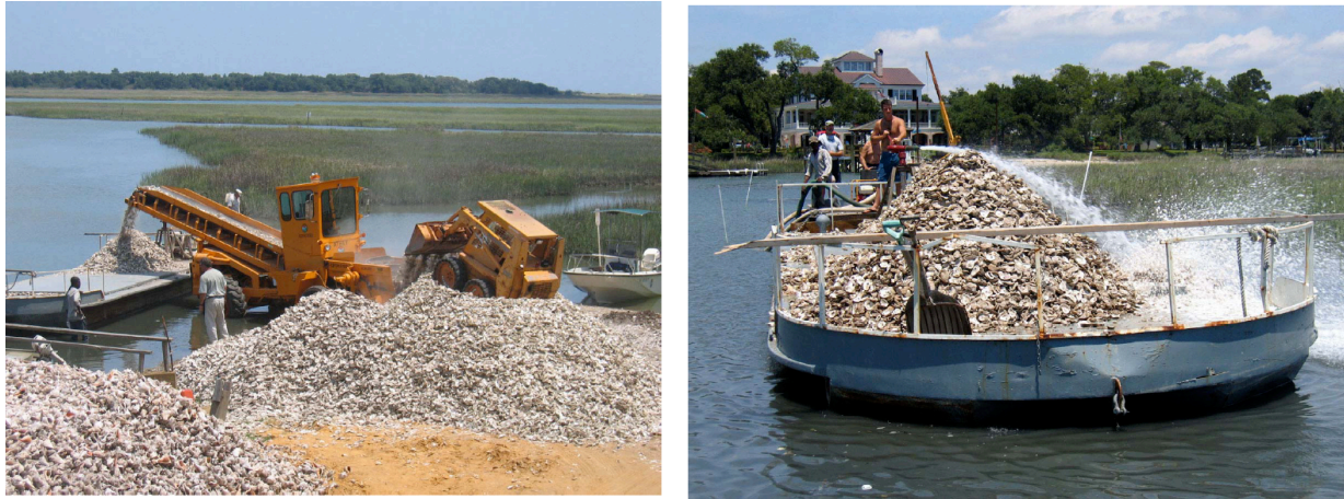
Figure 3. DNR equipment loads shell aboard a contractor's barge (left). High pressure water is used to blow the shells onto the shoreline (right).
