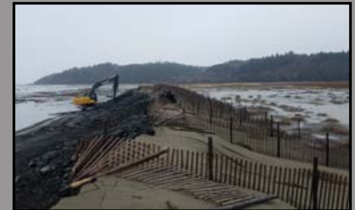
Crews reinforce the Shoalwater Bay dune barrier in response to an emergency declaration to protect the town of Tokeland.
