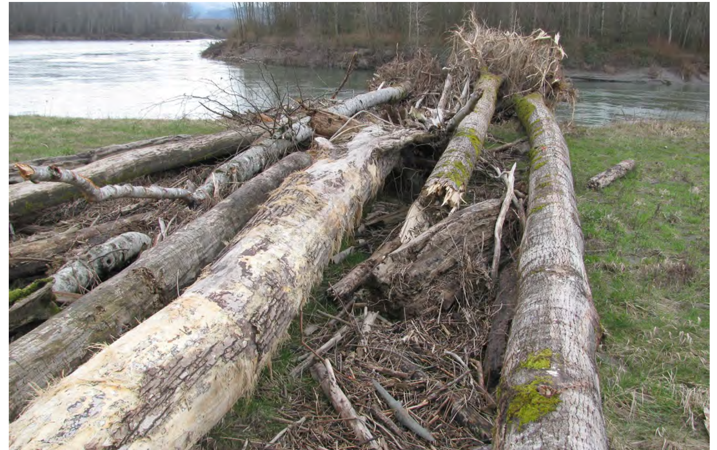
Above: Large logs with rootwads were laid on the riverbed bench of the levee as a mitigation feature that delivers benefits to the fish during high river flows. Skagit River has been designated as a critical habitat for three salmonid species listed under the Endangered Species Act. (USACE photo)
