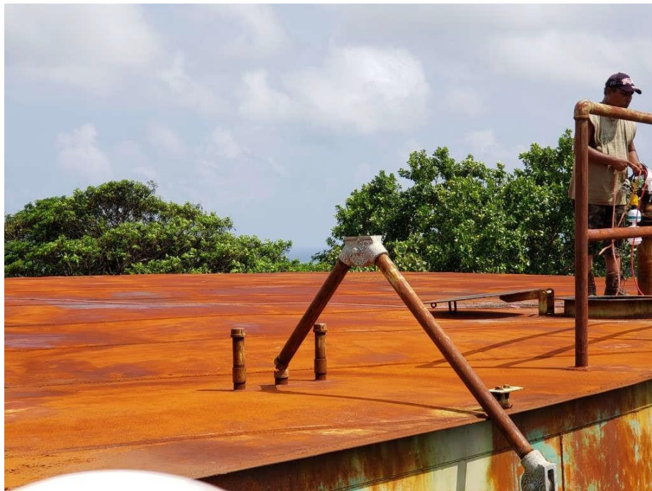
Photo D Damaged Level Gauge
