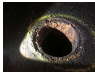
Under Bottom Suction Weld Corrosion
