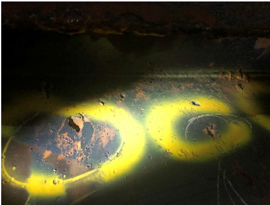
Photo D Typical Shell Plate Pitting
