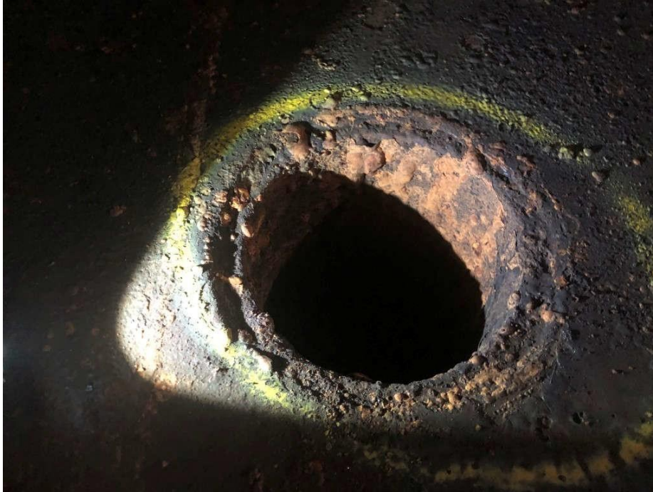
Photo J2 Under Bottom Suction Weld Corrosion
