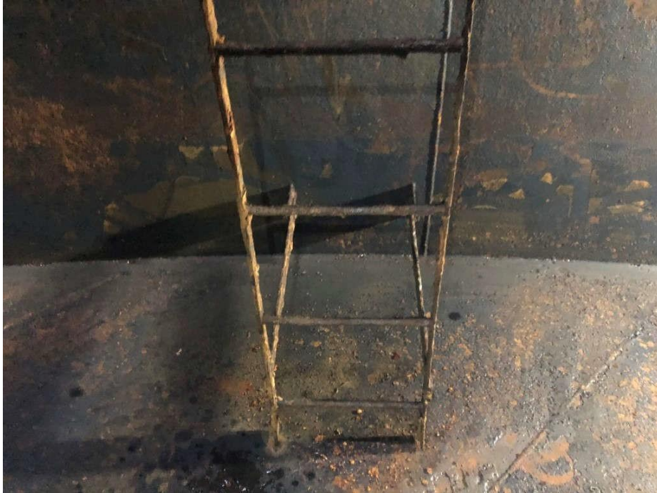
Photo I Corroded Internal Ladder
