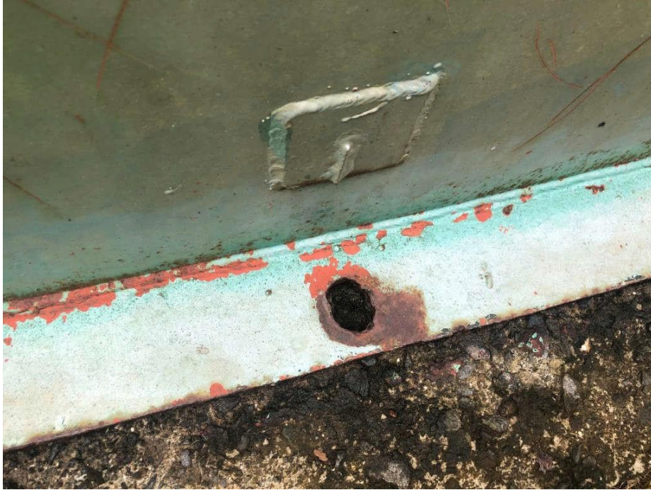
Photo N Missing Anchor Bolt
