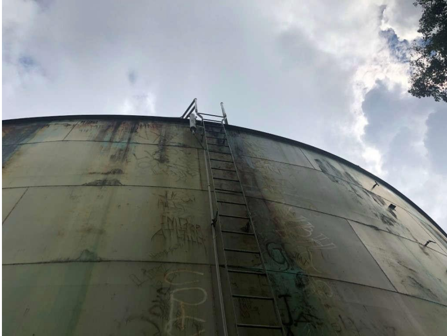
Photo L No Fall Restrain System on Vertical Ladder
