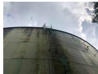
No Fall Restrain System on Vertical Ladder
