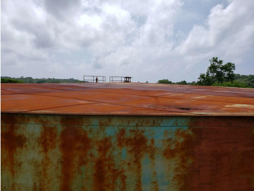
Photo F Through-Hole Corrosion on Roof
