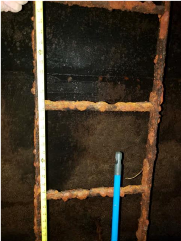
Photo B Corroded Internal Vertical Ladder
