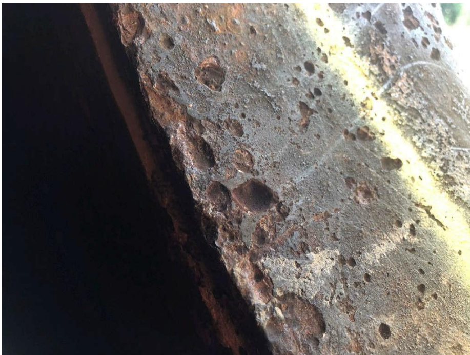
Photo H Pitting on Manway Neck
