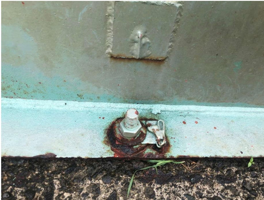
Photo G Typical Cathodic Protection Disconnection
