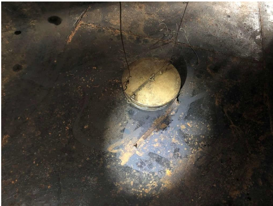
Photo M Level Float Disconnected
