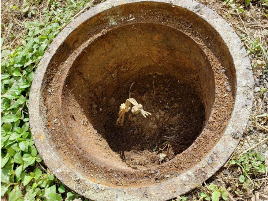
Photo A Disconnected Cathodic Protection
