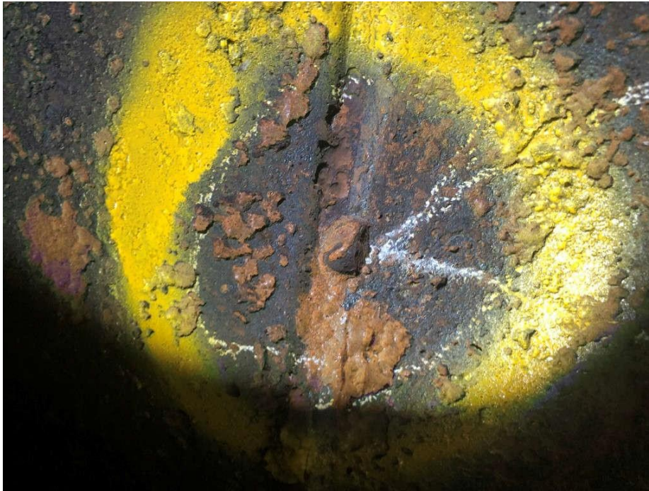
Photo C Typical Vertical Weld Pitting
