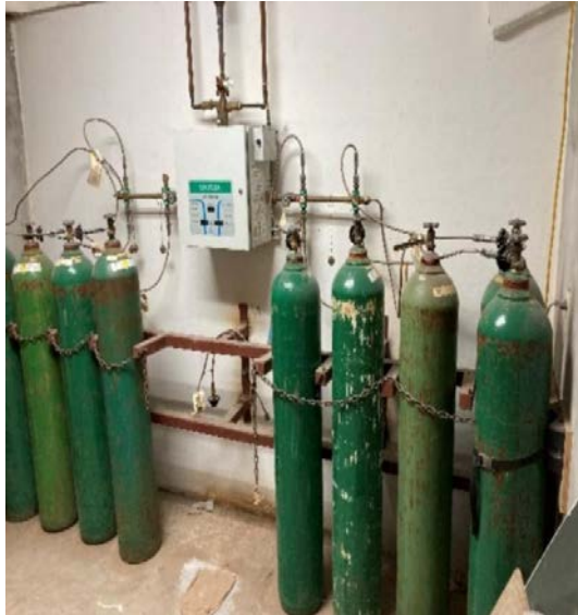
Installed Oxygen Manifold
