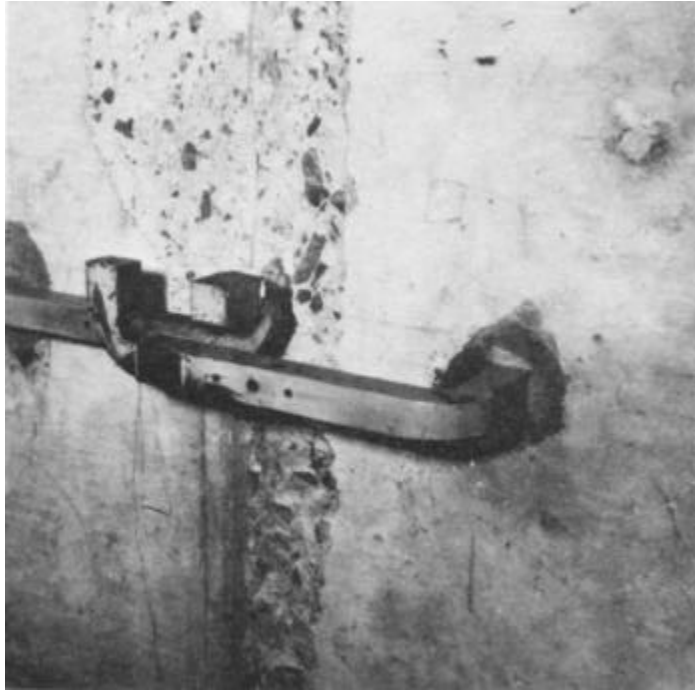
Figure 5-1. Monolith Joint Displacement Indicator. (Photo by WES)
