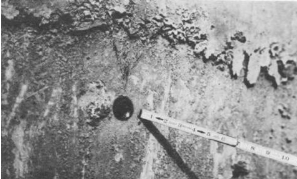
Figure C-13. Embedded Joint Meter Socket with Plug Removed (Courtesy of the Tennessee Valley Authority).
