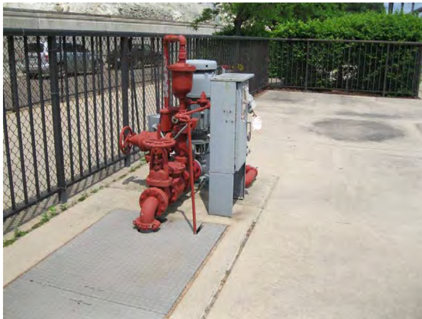
Figure 10-49. Fire pump system mounted on the lock wall
