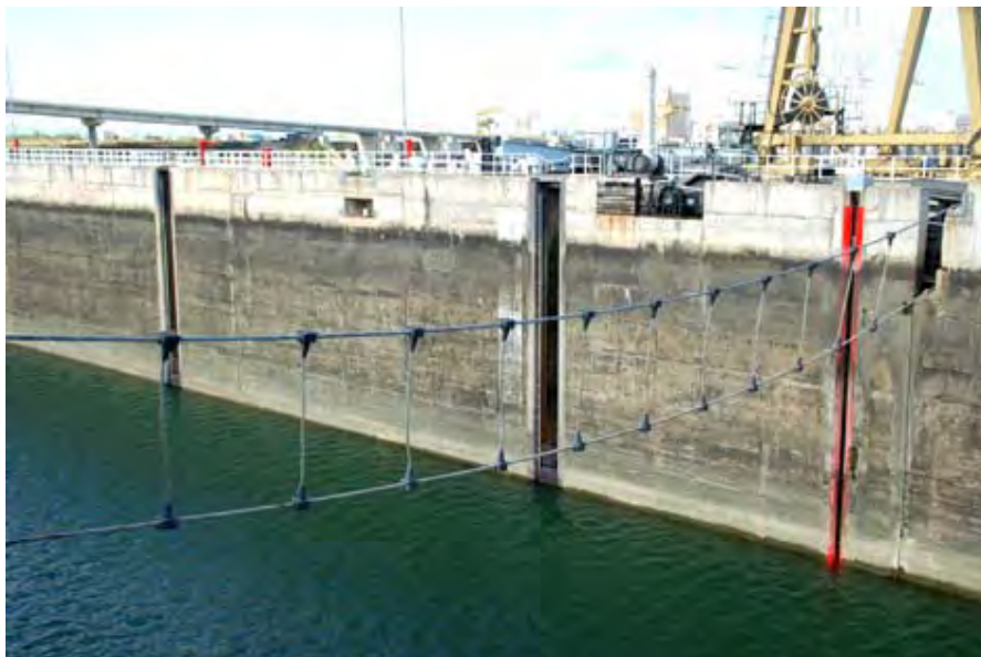
Figure 10-36. Gate protection structure: steel wire ropes across the lock chamber
