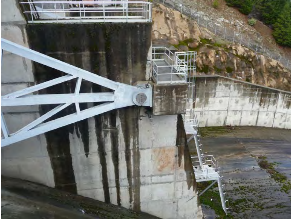
Figure 9-3. Tainter gate trunnion bearing
