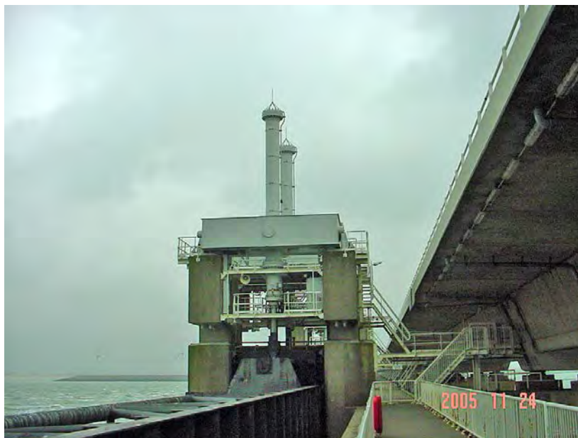
Figure 7-7. Direct-connected hydraulic vertical storm gate
