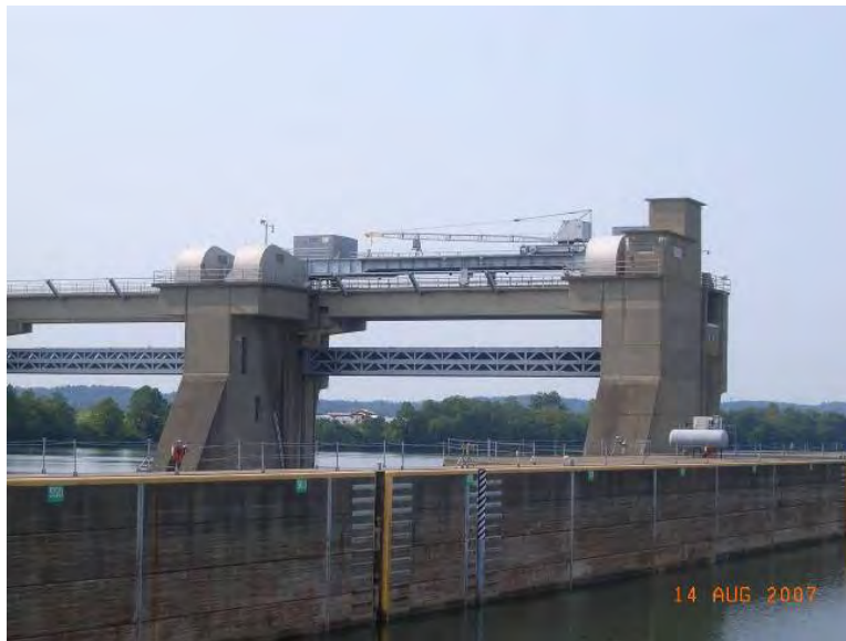
Figure 10-43. Bulkhead crane with auxiliary piggyback crane, Racine Dam, Ohio River, one bulkhead section is stored in each gate bay
