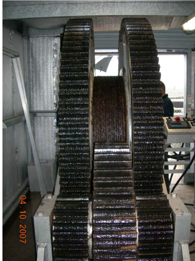
Figure 10-47. Lowering carriage machinery, Port Allen Lock
