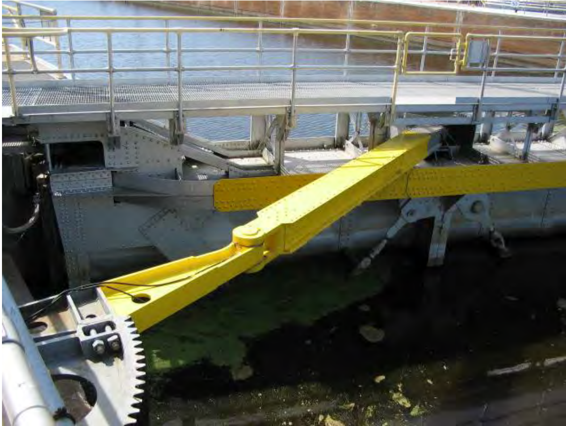
Figure 4-11. Miter gate strut arm
