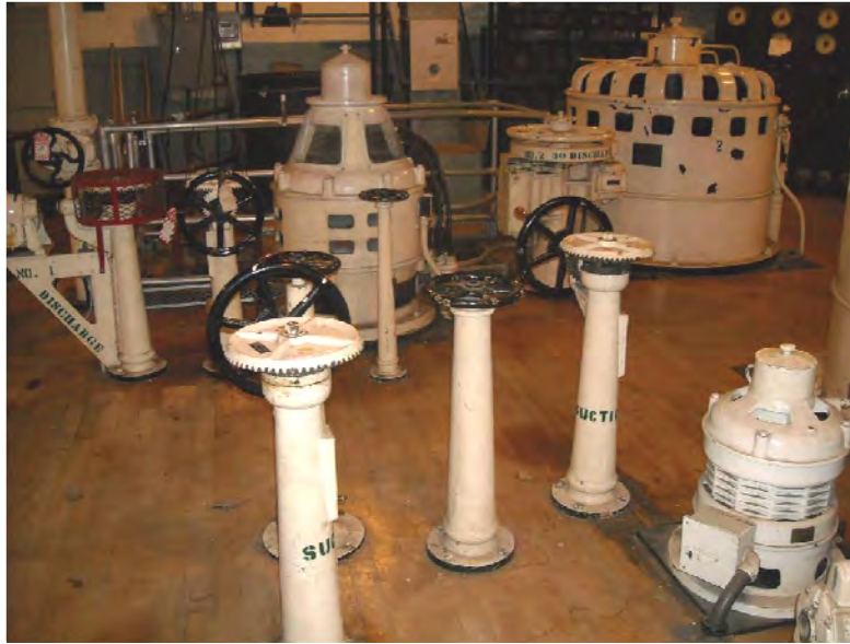
Figure 10-24. Dewatering pumps and valves, Chittendon Locks, USACE
