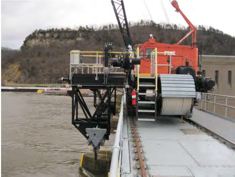
Figure 10-42. Maintenance crane installed on undercarriage
