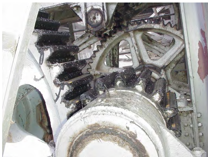
Figure 2-28. Greased open gear set
