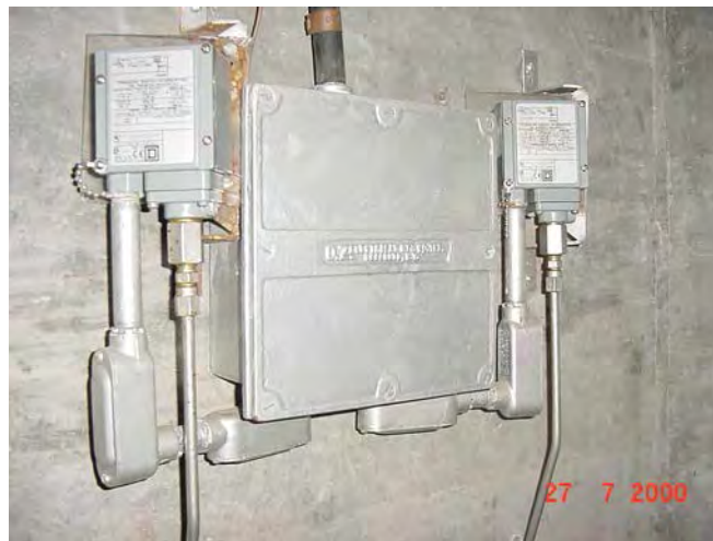
Figure 2-25. Hydraulic pressure limit switch
