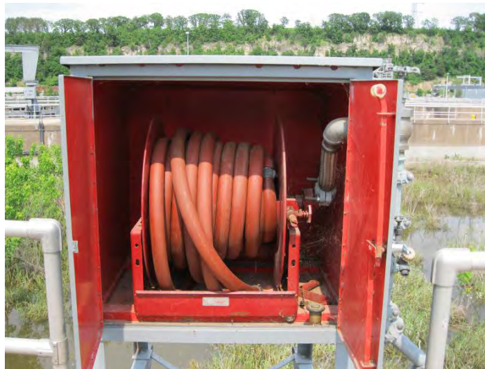
Figure 10-52. Hose reel mounted inside cabinet
