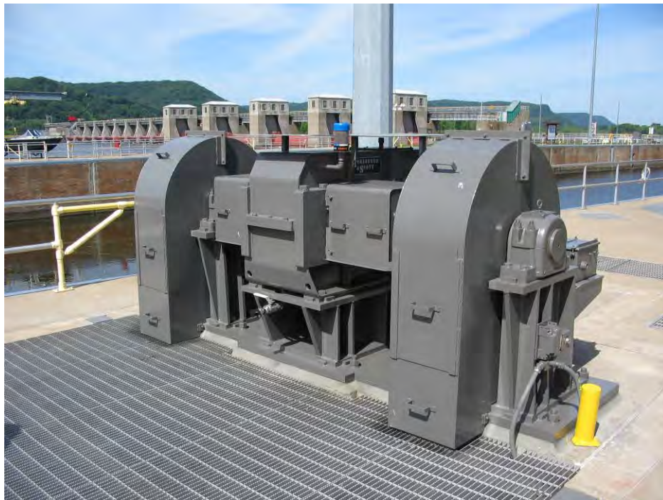
Figure 6-2. Electric Motor Driven Tainter Valve Hoist
