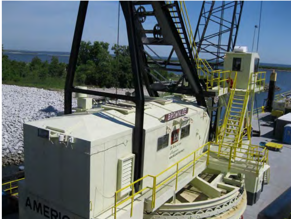
Figure 10-39. Barge-mounted crane for maintenance and repair
