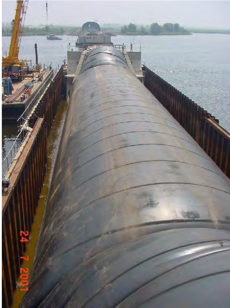
Figure 9-27. Ramspol storm surge protection bladder dam (courtesy of R.A. Daniel, Rijkswaterstaat, Division of Infrastructure, Netherlands)
