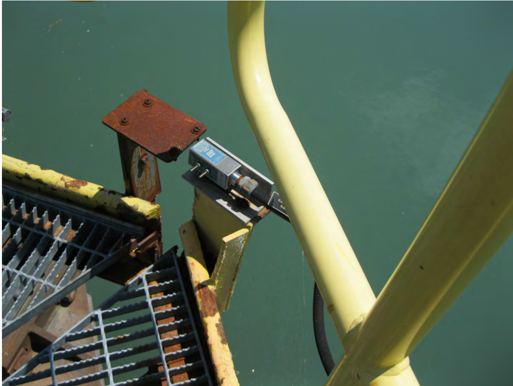
Figure 4-14. Miter gate position limit switch
