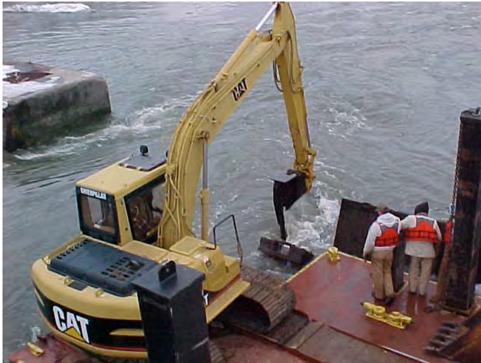
Figure 9-14. Modified excavator operating manual wicket gates
