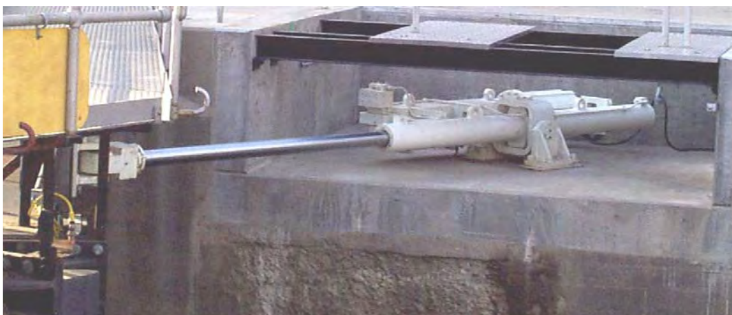
Figure 4-10. Self-contained actuator – US Army Corps of Engineers Pittsburgh District
