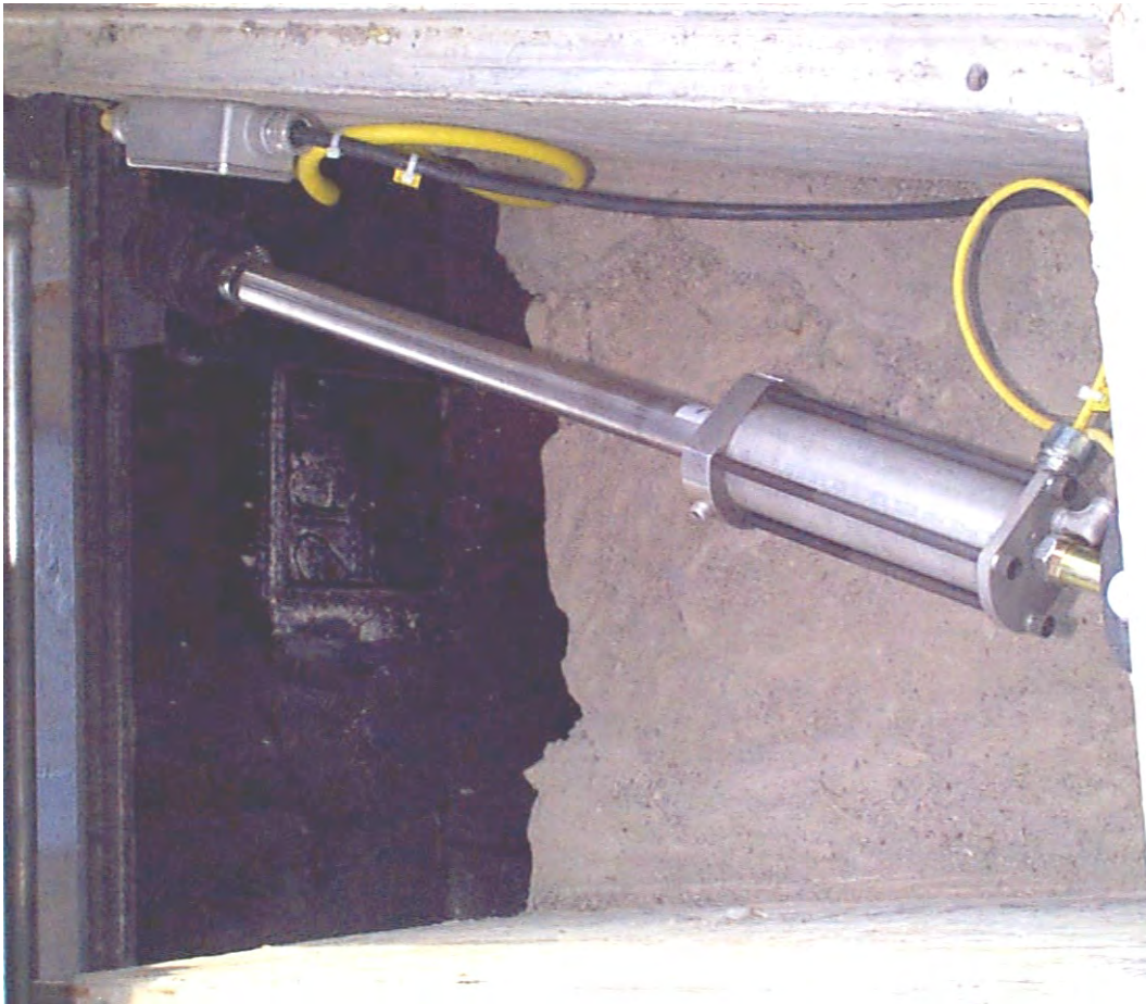
Figure 3-5. Small LDT enclosed in cylinder-type housing and attached to miter gate near the gudgeon pin
