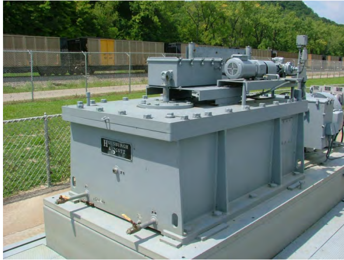
Figure 2-42. Miter gate speed reducer
