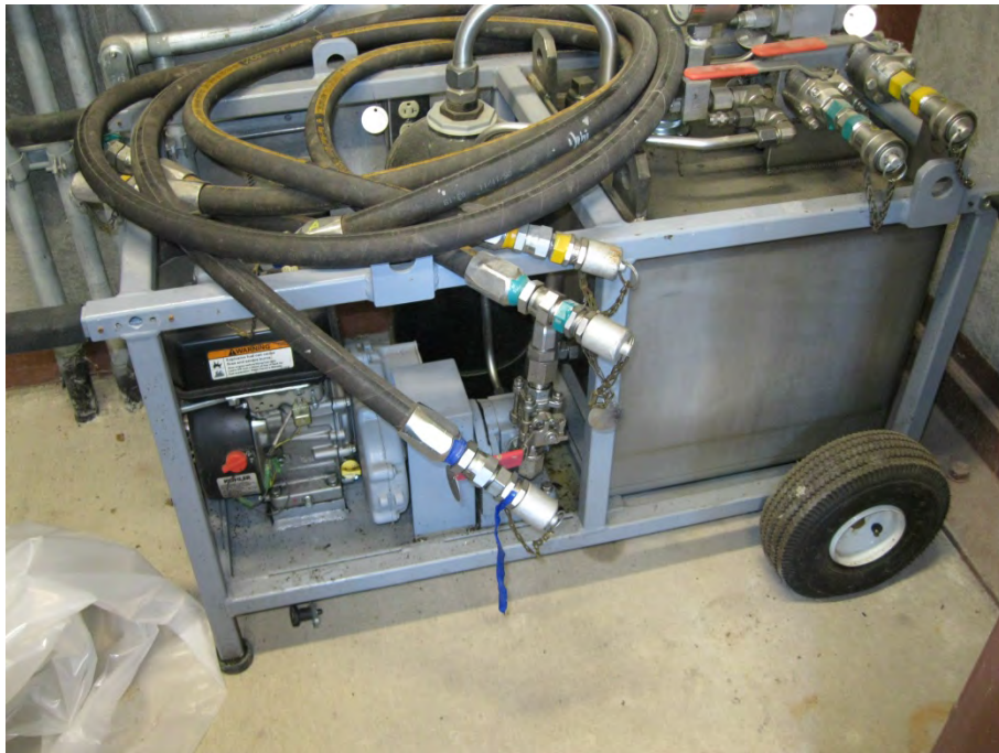
Figure 5-5. Auxiliary power unit for Bayou Dupre Gate, New Orleans
