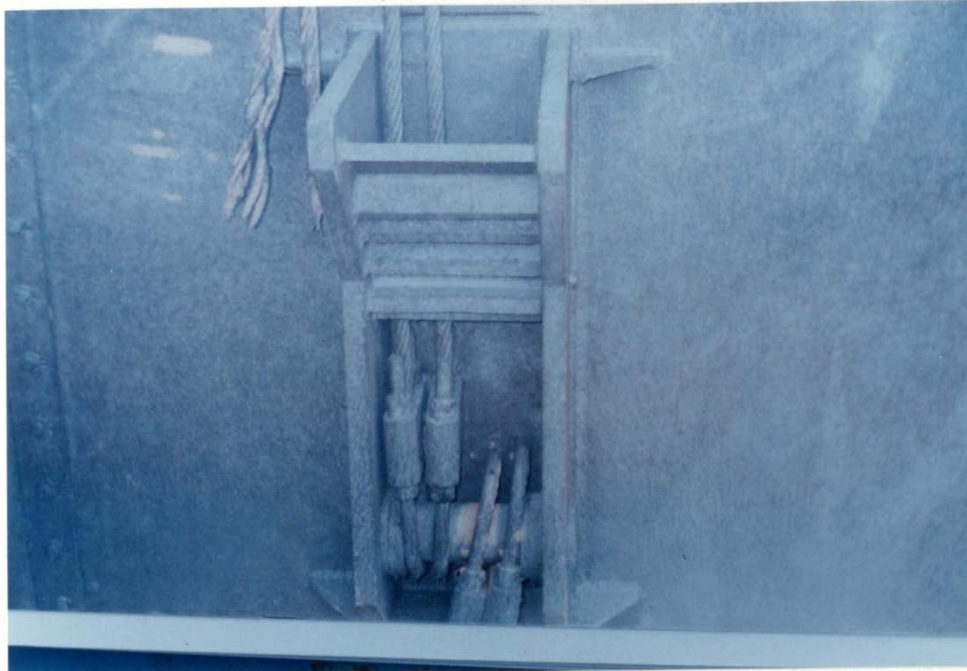
Note the broken cables.
