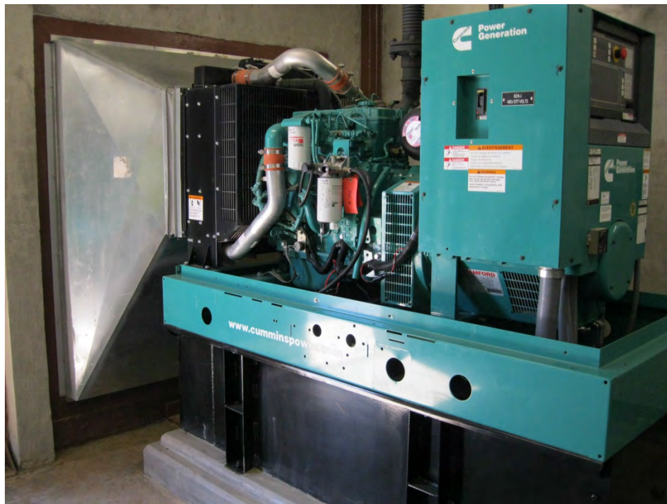
Figure 5-6. Bayou Dupre, New Orleans, backup generator
