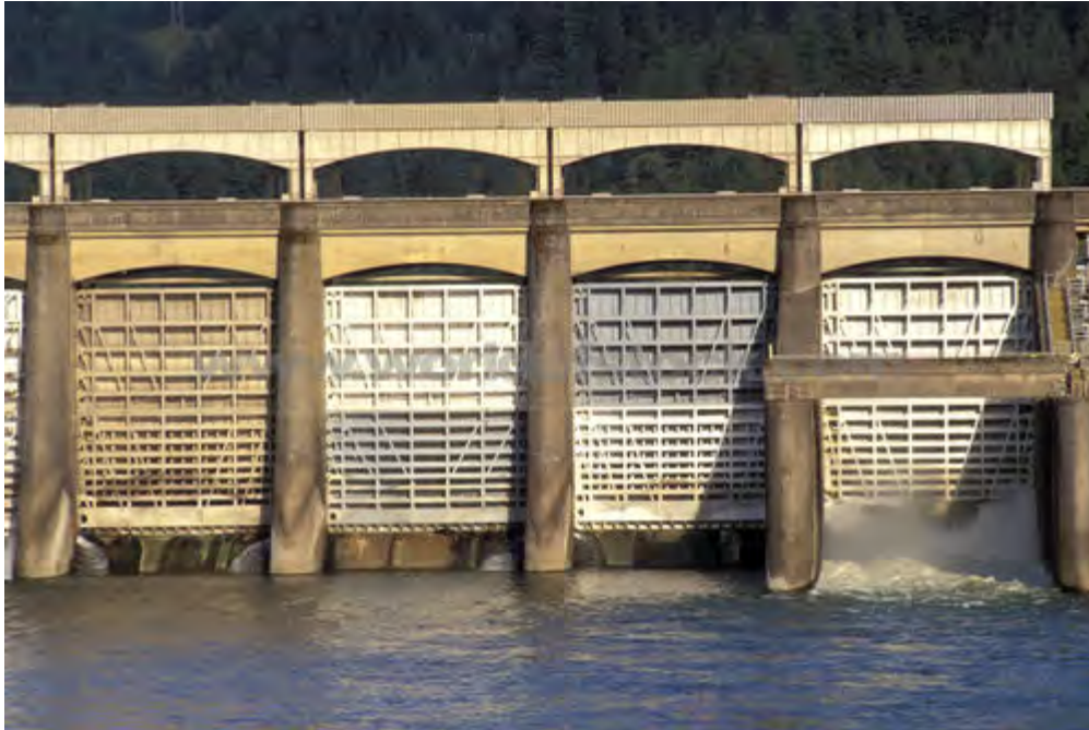
Figure 9-12. Spillway vertical lift gates
