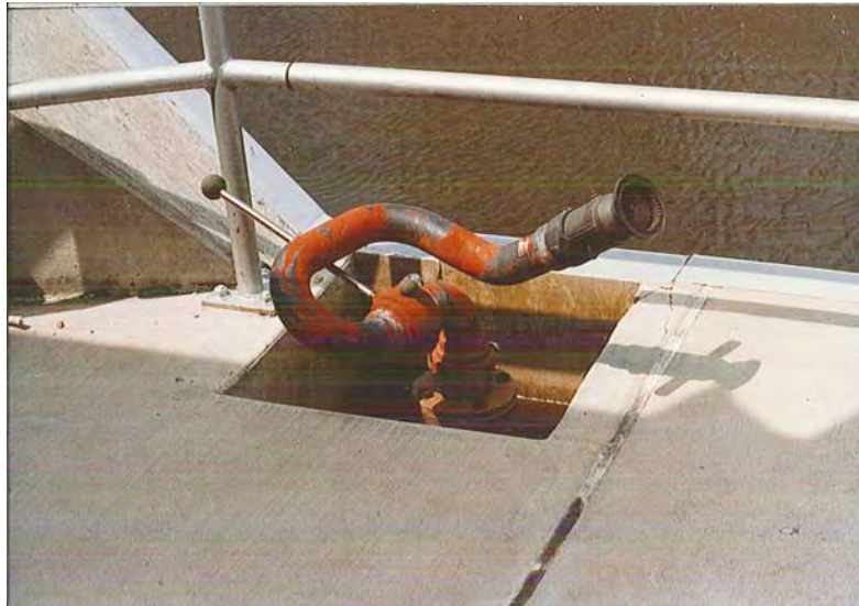
Figure 10-50. Spray nozzle mounted on lock wall
