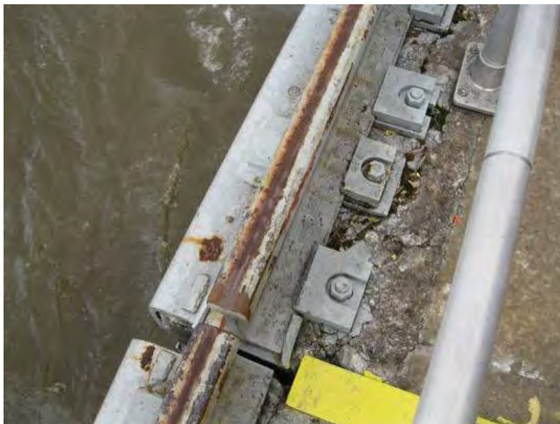
Figure 10-6. Gaps in rail section of travelling keel
