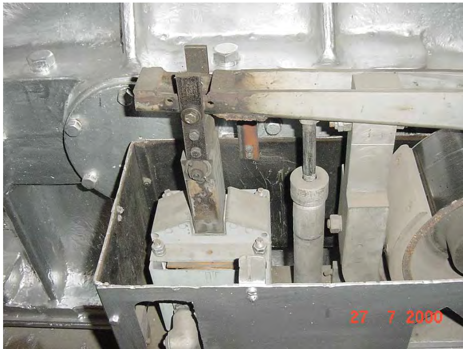
Figure 2-17. AC rectified brake
