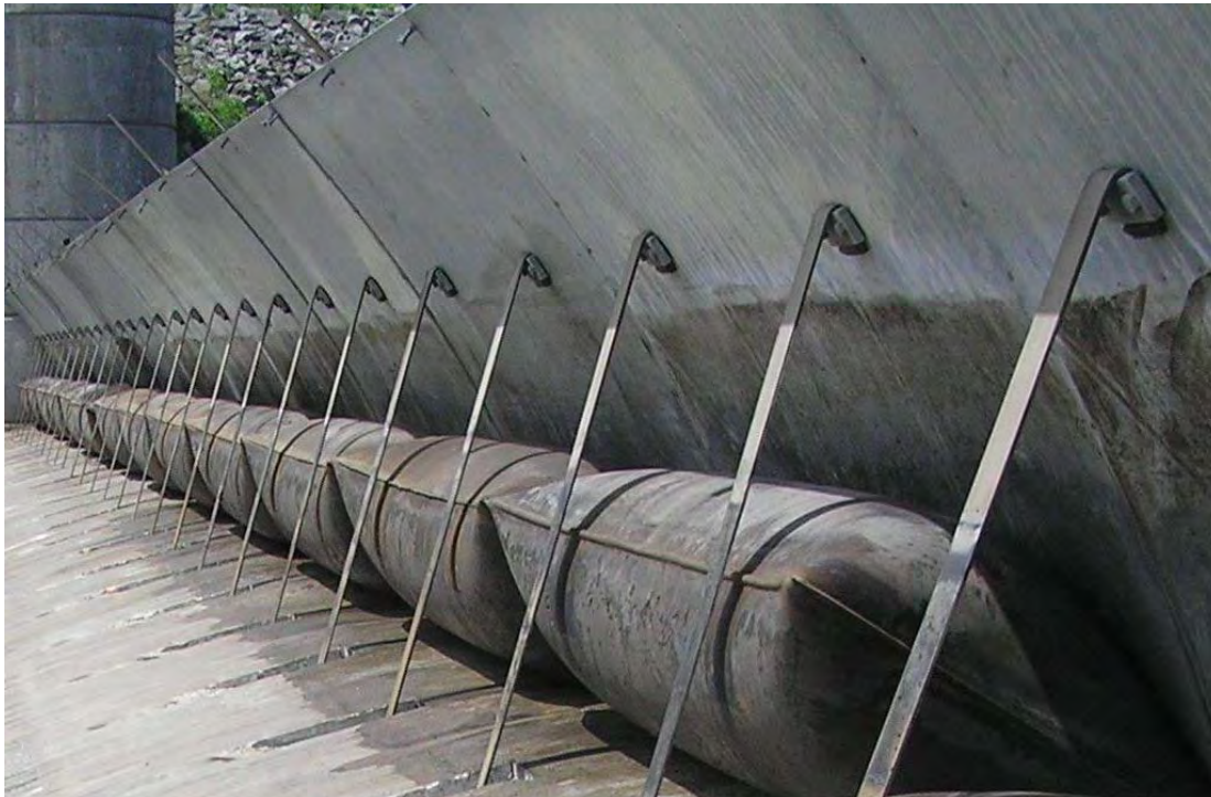
Figure 9-22. Inflated air bladder below closed hinged crest gate
