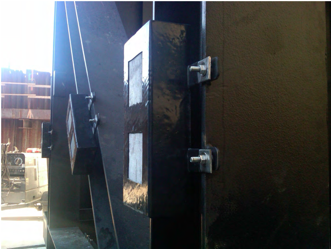
Figure 10-53. Sacrificial anodes installed on a sector gate, New Orleans
