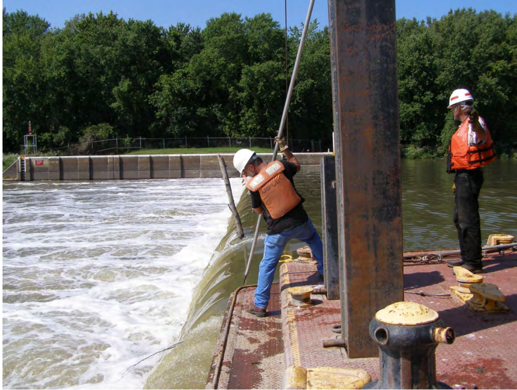
Figure 9-15. Raising manual wicket gates
