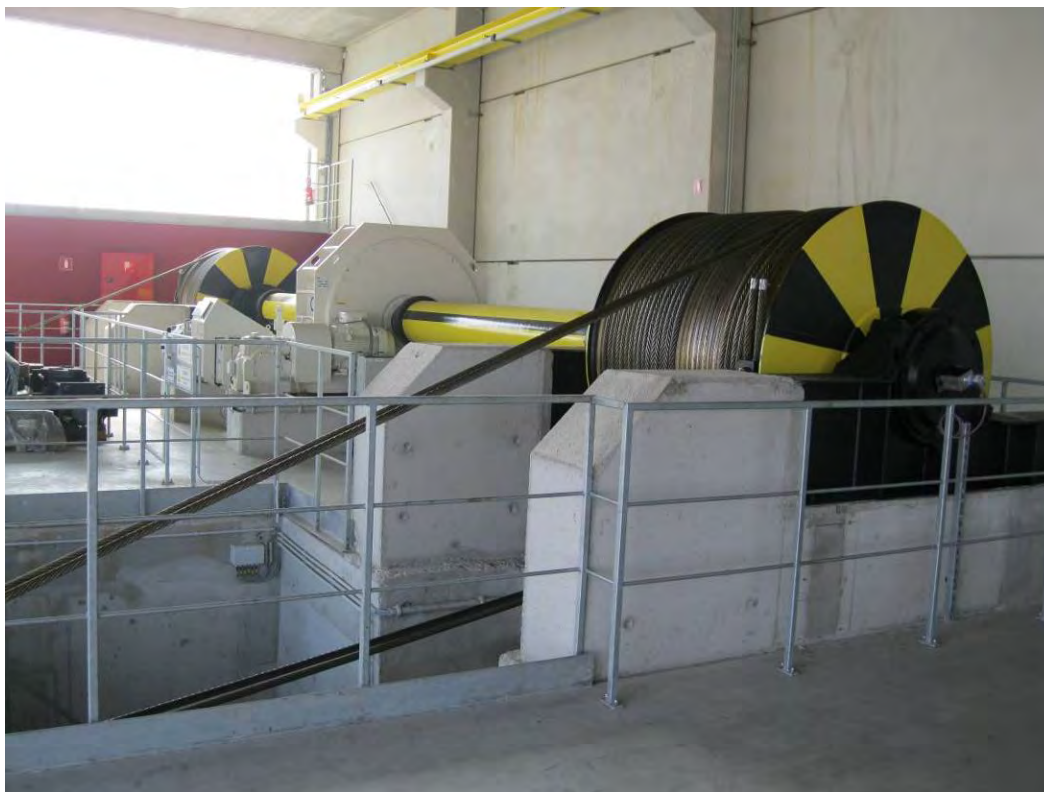
Figure 8-5. Rolling gate machinery, Van Cauwelaert Lock, Antwerp, Belgium
