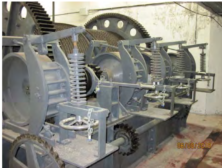
Figure 10-33. Energy absorption cable drum, St. Lawrence Seaway
