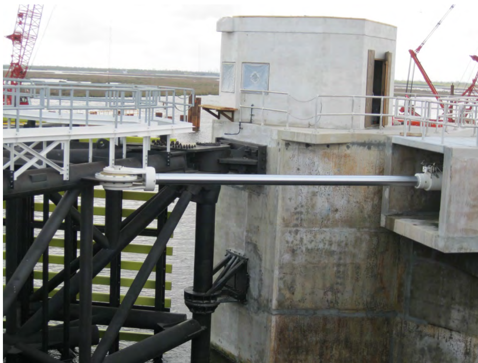
Figure 5-3. Hydraulic cylinder-driven sector gate, New Orleans
