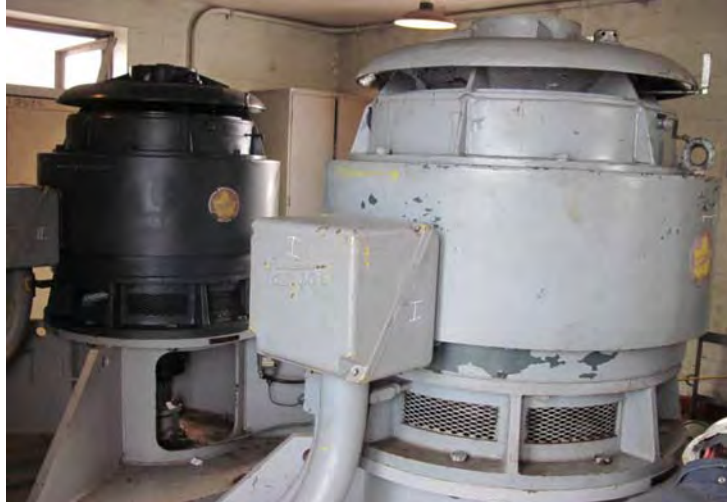
Figure 10-22. Vertical pump motors, St. Lawrence Seaway
