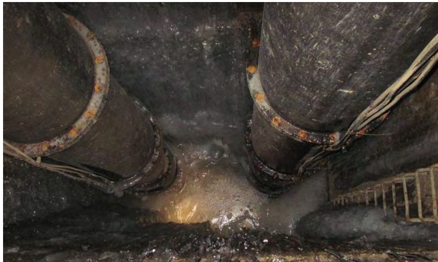
Figure 10-21. Vertical pumps, St. Lawrence Seaway
