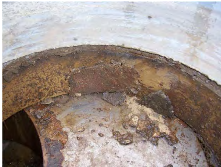
Figure 2-4. Failed gudgeon pin bushing
