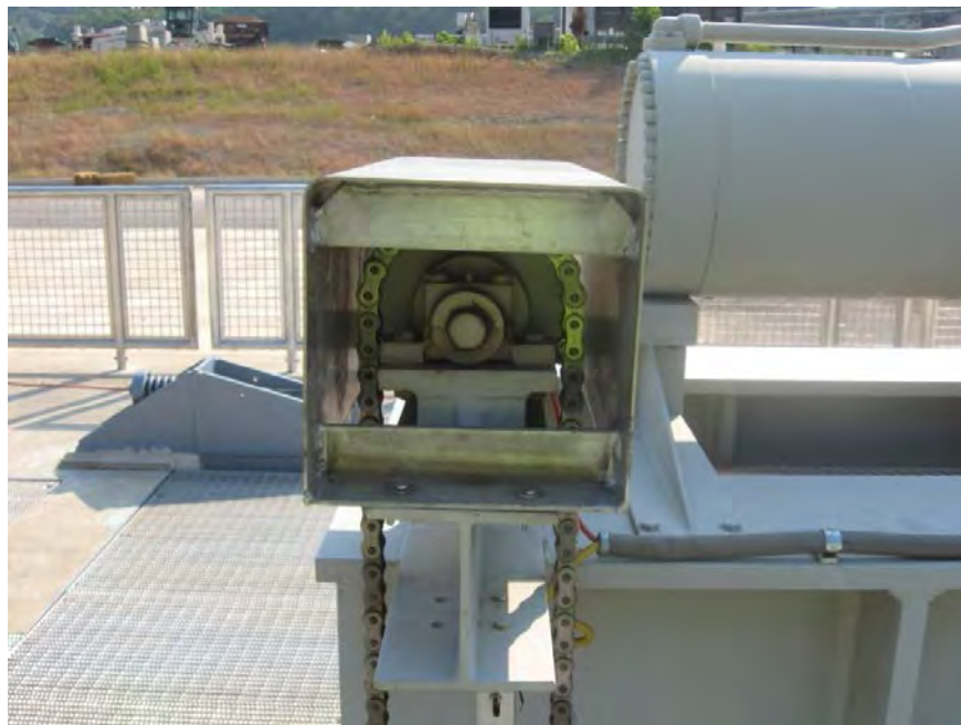
Figure 3-3. Position encoder driven by roller chain connected to stoney gate valve
