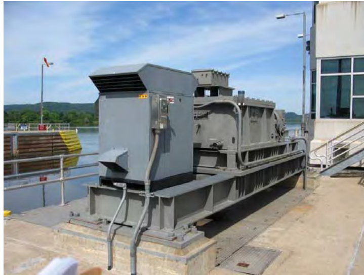
Figure 10-8. Localized compressor installed on miter gate machinery
