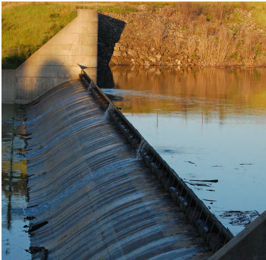
Figure 9-21. Air bladder-operated hinged crest gate
