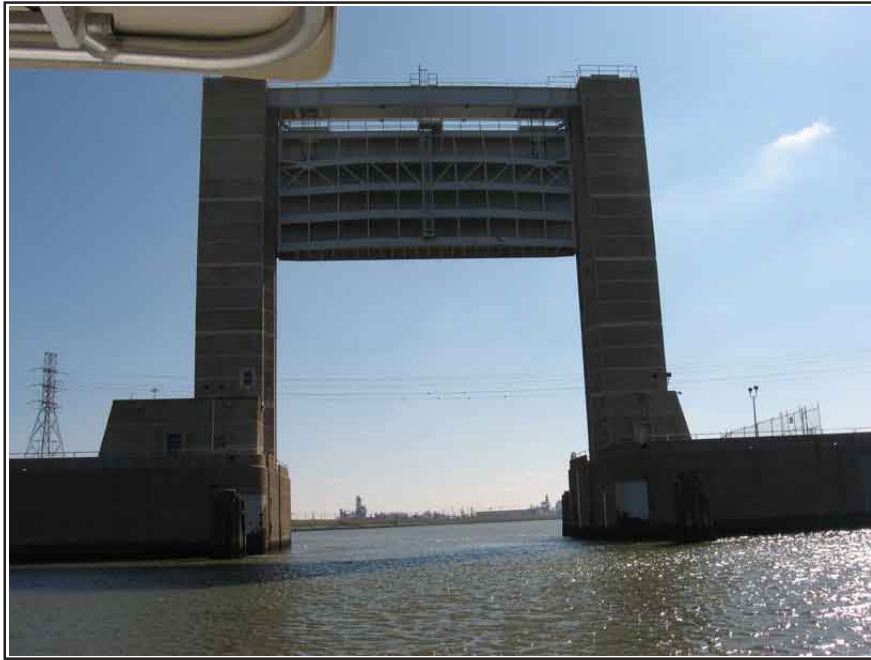
Photo 1 - View of flood control gate located at the northern extent of the project area at the Stauffer Turning Basin, facing northwest.
