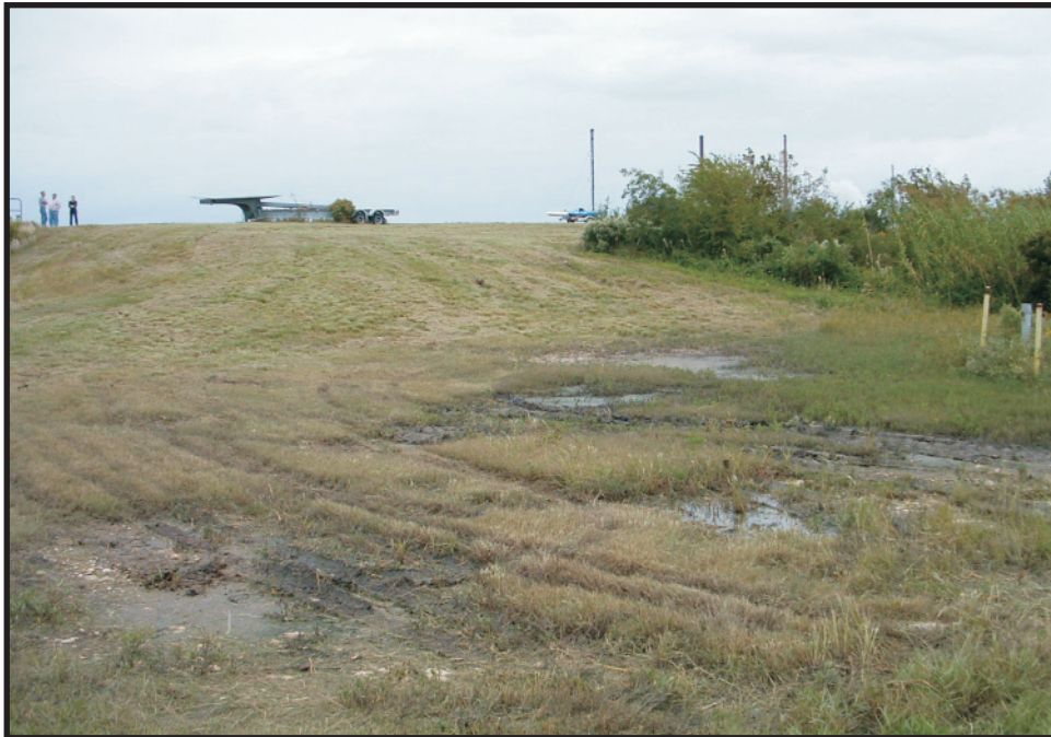
PHOTO 14 Area south of levee on east bank of Alligator Bayou, facing north
