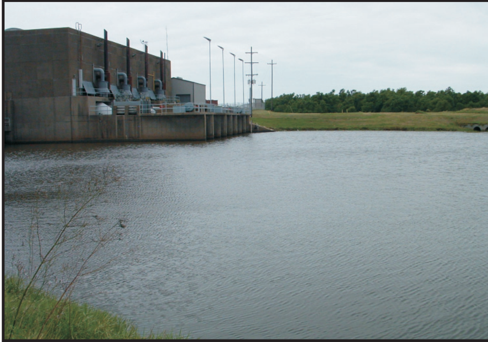
PHOTO 11 View of existing intake pumps, facing west
