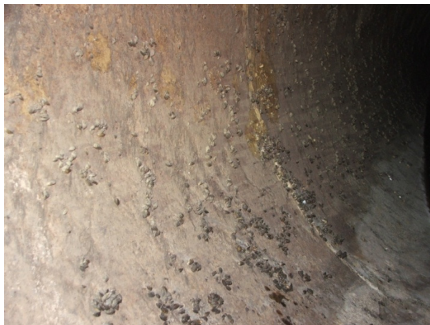
Figure 2-7 Zebra Mussels Attached to a Pipeline
