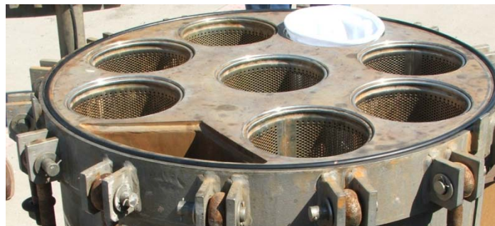
Figure 10-2- Housing of a Bag filter Unit
