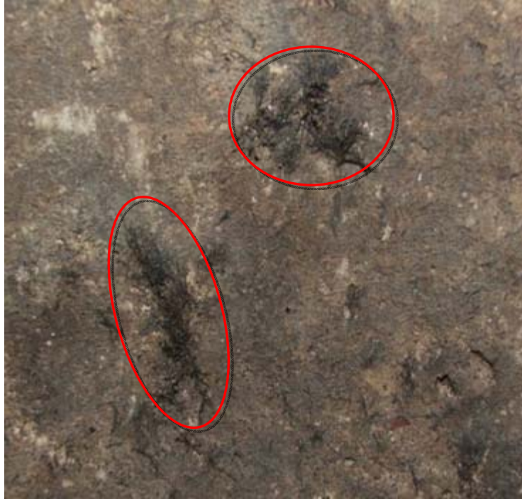
Figure 2-4- Byssal Threads Remaining on a Concrete Pipe Wall
