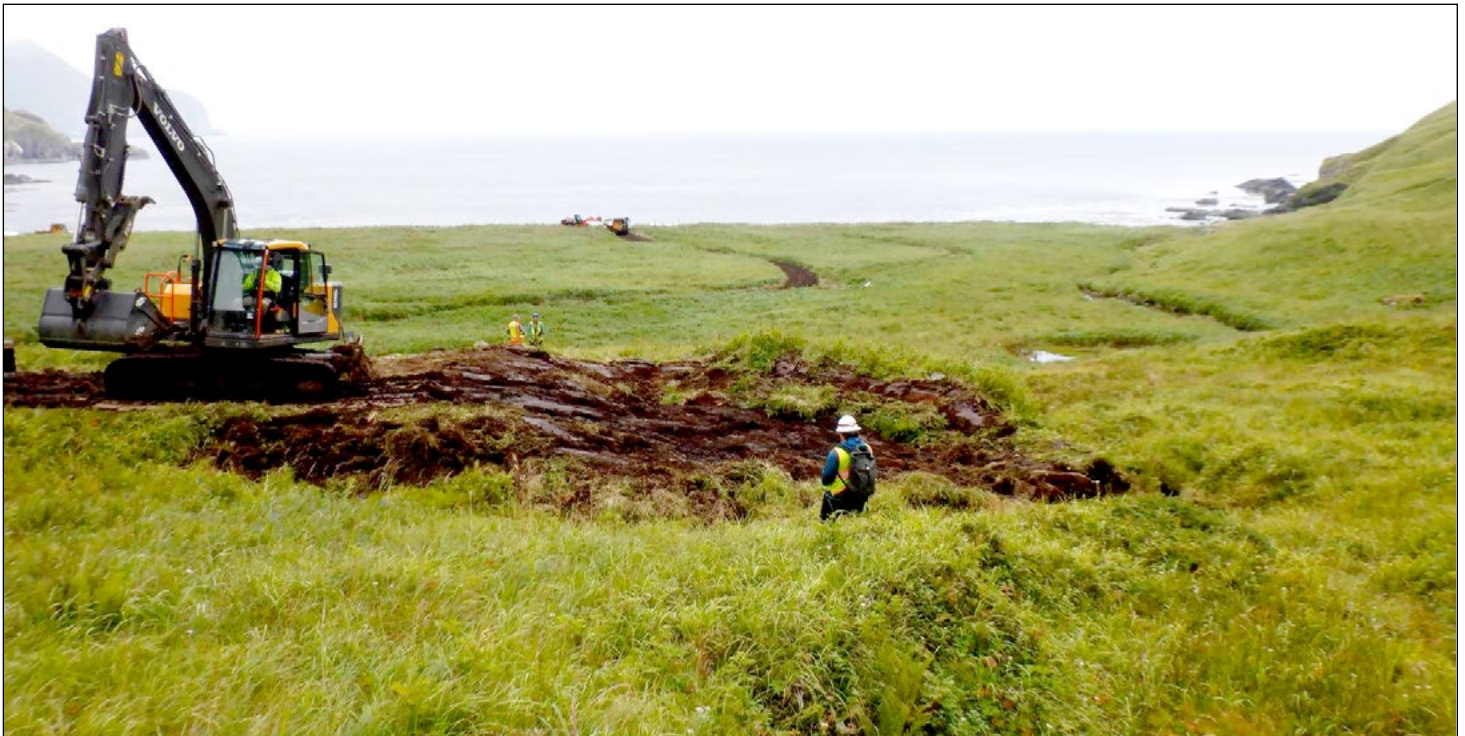
Crews work to recontour excavated areas to match the surrounding topography and replace the organic layer at the Cape Prominence Formerly Used Defense Site.
