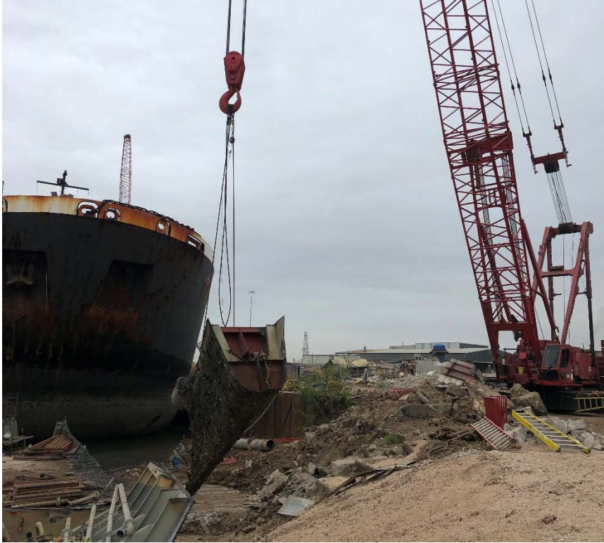
The final section of the vessel is removed from the water and placed on the dock for sectioning into smaller pieces to be made available for recycling.
