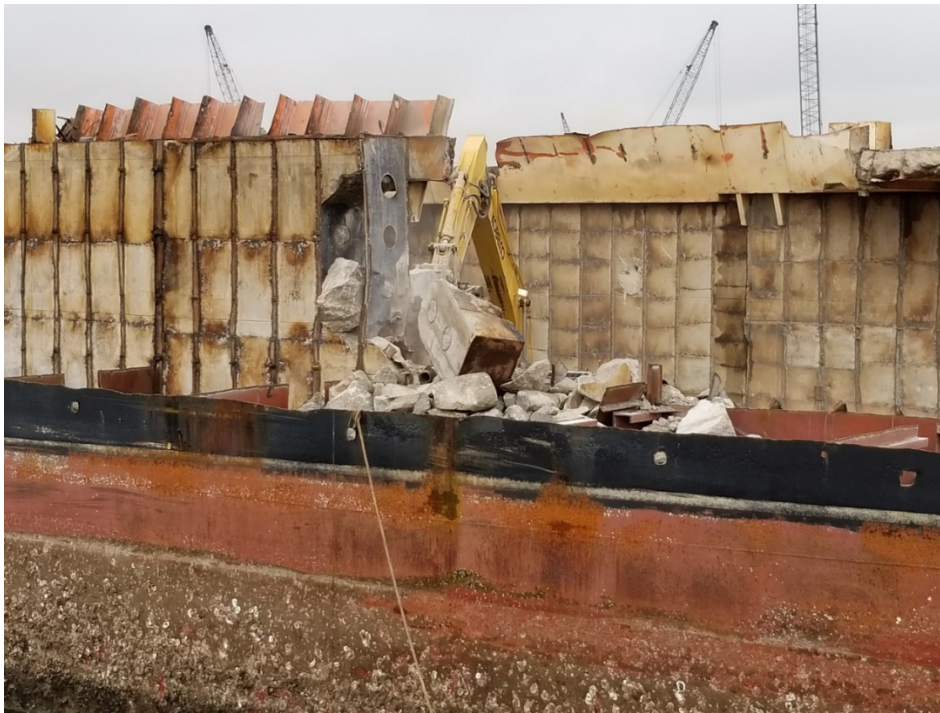
Dismantlement of the collision barrier on the STURGIS barge. The collision barrier was designed to protect the reactor components in the event of a collision when the STURGIS and the MH-1A reactor were operational.
