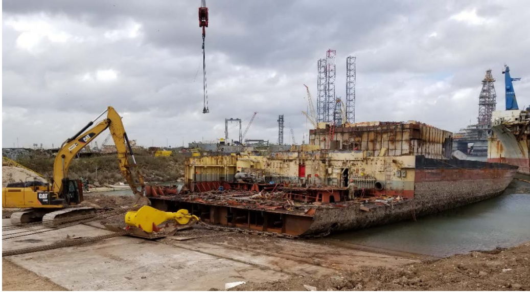
View from stern looking forward toward bow during shipbreaking of STURGIS in February. Crews are cutting the vessel into sections from stern to bow and moving it further ashore as progress is made.
