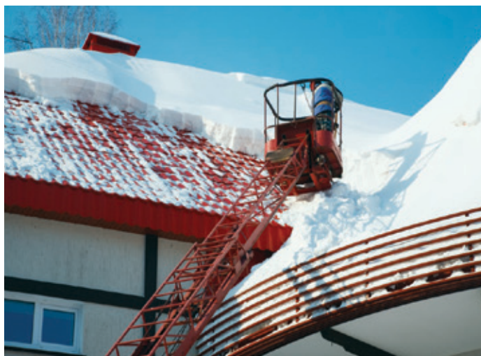
An aerial lift is being used in a snow removal operation. The worker is using a restraining belt and lanyard for protection.
