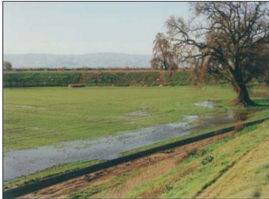
Figure 2-9: Areas of Seepage 1997, RD-17 ( \approx RM 8.5)
