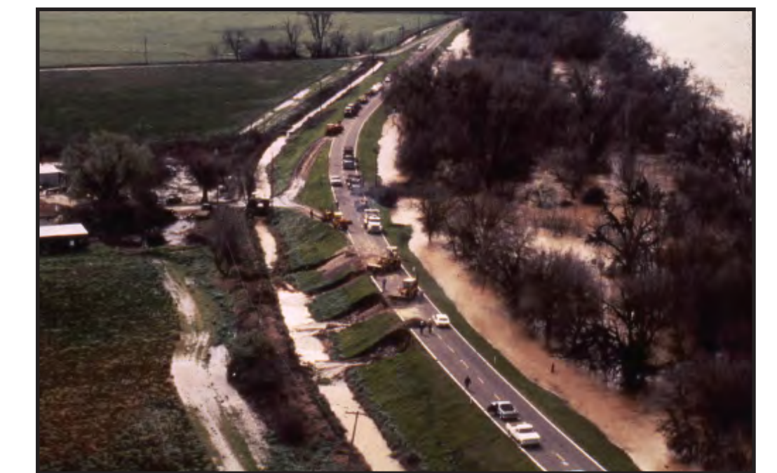
Seepage and stability problems
