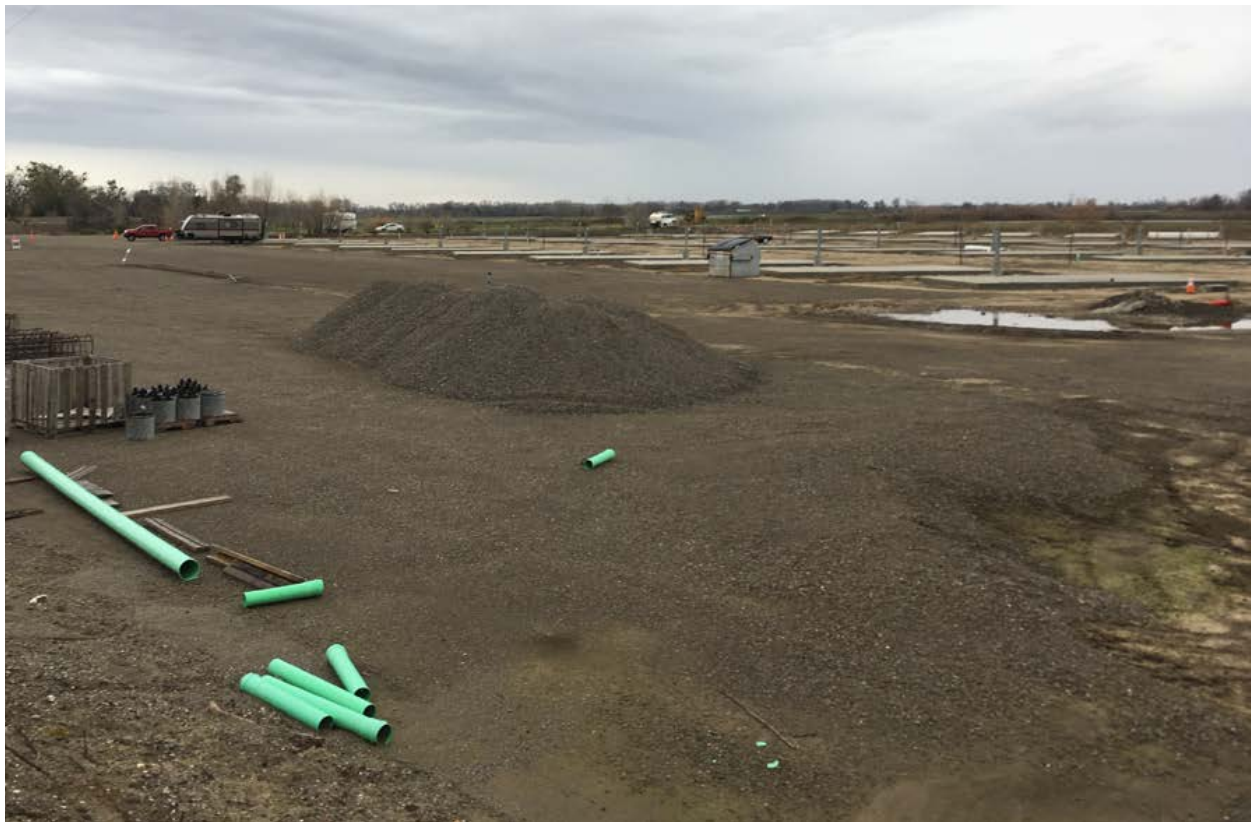
Figure 2. Site photograph taken by U.S. Army Corps of Engineers biologist on February 25, 2019.
