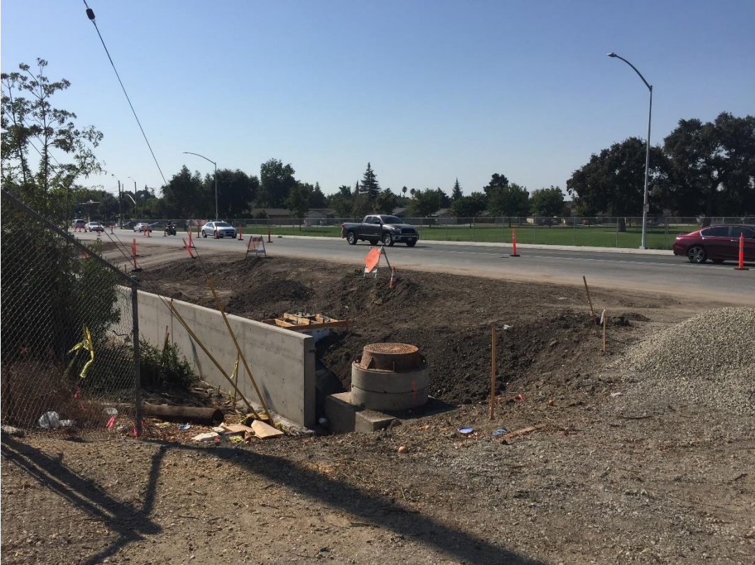
Thornton Road Widening Project Conform Work at Bear Creek (Southeast Side of Bear Creek Bridge on Thornton Road).
