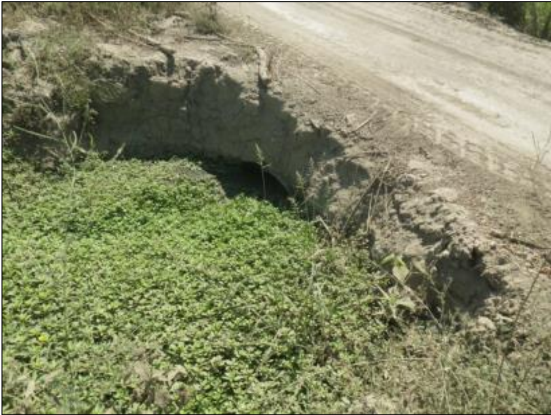
Photo 4. View of upstream, northern face of Agricultural Road Crossing 2 (looking south) showing excessive vegetation build-up clogging an undersized culvert.
