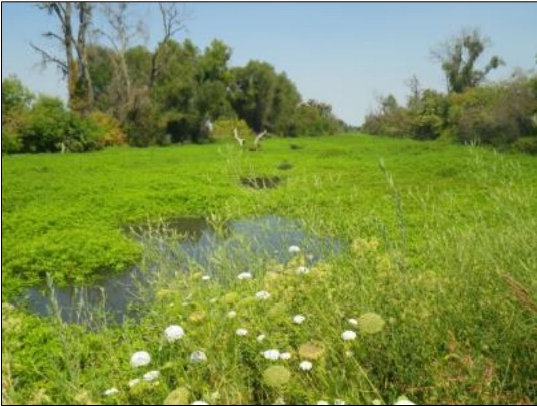
Photo 7. View upstream of Agricultural Road Crossing 3, showing vegetation growth concealing an undersized culvert looking north on road crossing.
