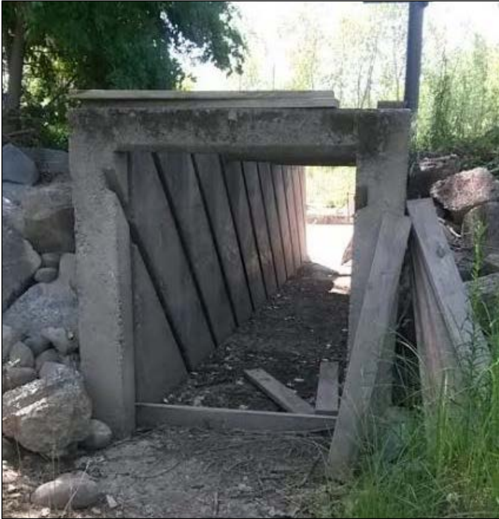
Photo 1. View of Existing Denil-type Fish Ladder with Stoplogs and Interior Baffles Removed, Looking Downstream.
