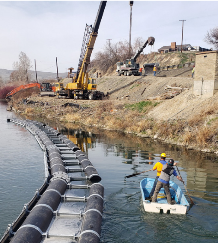
Sunnyside Valley Irrigation District crews installing the fish guidance boom in spring 2021.
