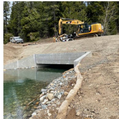
Davis Creek concrete box culvert installed under Boat Launch Road to allow fish passage.
