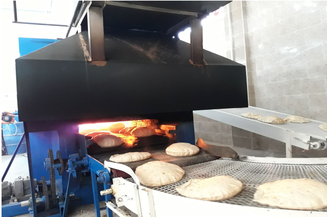
UNHCR in partnership with SIF installed a bakery production line. The bakery will cover 44,000 individuals with bread in 22 villages.
