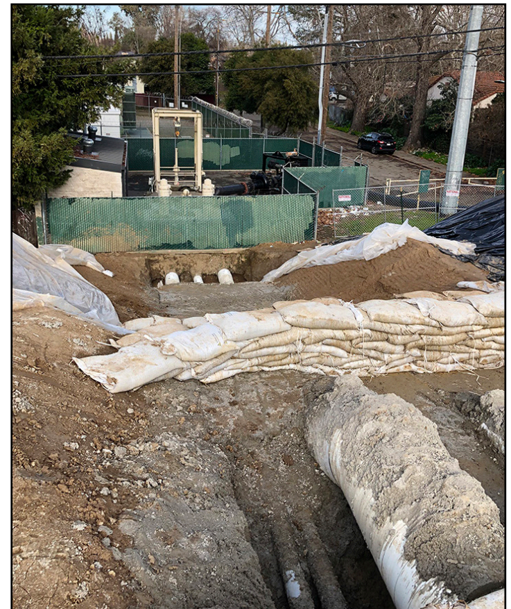
Discharge pipes run from City of Sacramento Sump 58 through the Garden Highway levee road. Garden Highway cannot be reopened until this pipework is complete.
