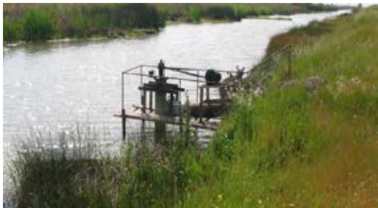
Figure 2: Typical Pump Station in PGCC
