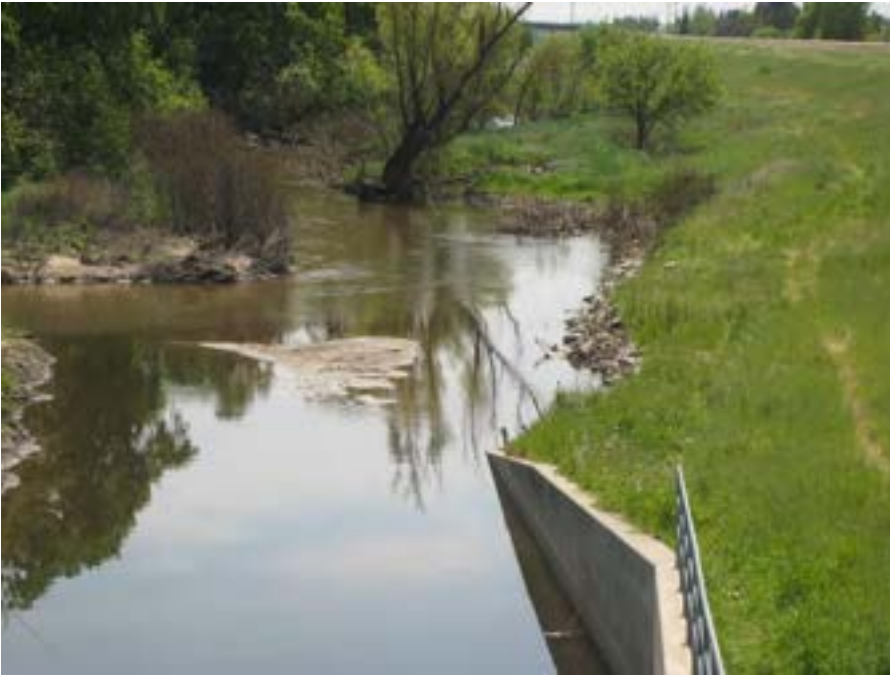
Photograph 3. NEMDC erosion site downstream of Pump Station 15
