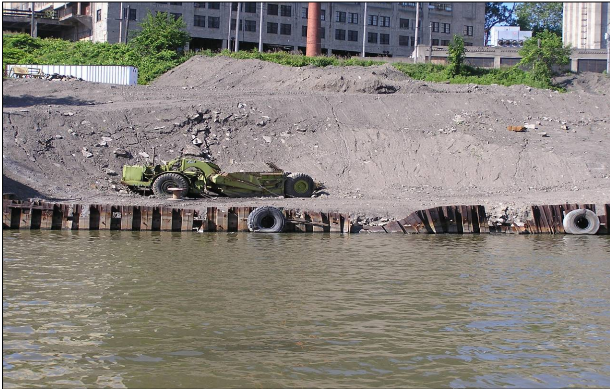
Figure 1.30 – Failed SSP bulkhead on the Cuyahoga River
